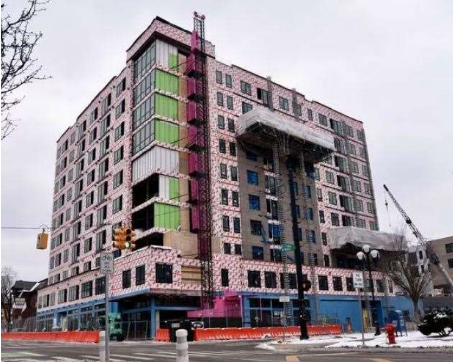
The Standard, Student Housing, Under Construction Recently In Ann Arbor (MLive; Rt Clk for Larger)
