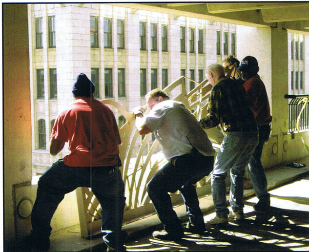
Staff from Republic Parking helping Irina Koukhanova remove a steel panel for repair.
