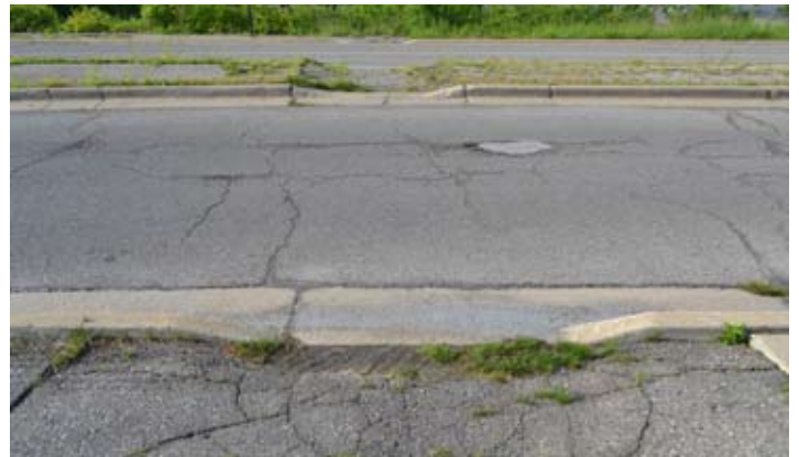
Sidewalks and pedestrian crosswalks are deteriorated
