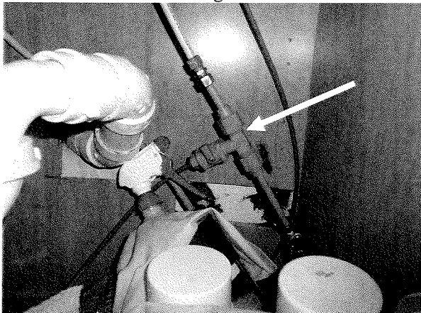
Polybutylene supply lines at sinks.
