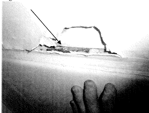
Second floor shower surround, with mold-like substance behind wall.
