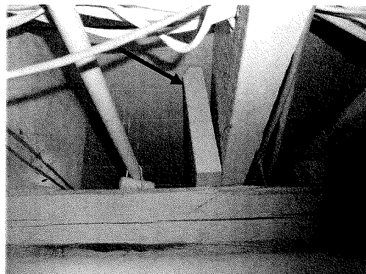
Basement joist "rolling"; not properly supported.
