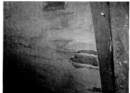
Spalling, deterioration of brick in central basement wall.
