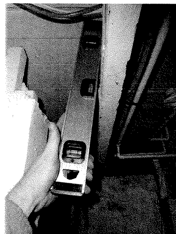
Basement joist cracked, rotated.
