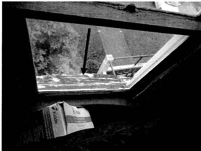
Window sills require maintenance.
