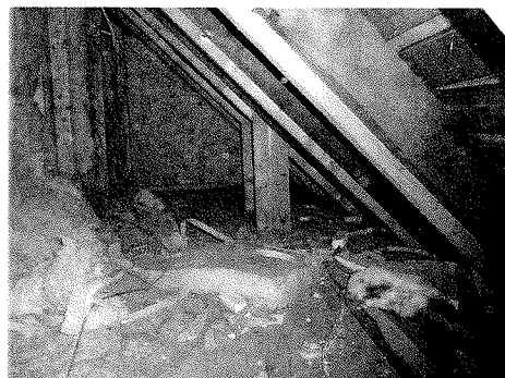
Displaced insulation in east attic, north.
