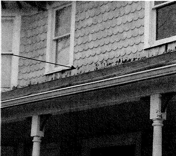
Siding over east porch damaged/rotted.
