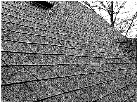
Roof showing signs of cupping/curling.
