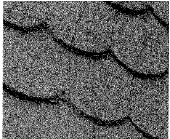
Scalloped siding requires maintenance/replacement.
