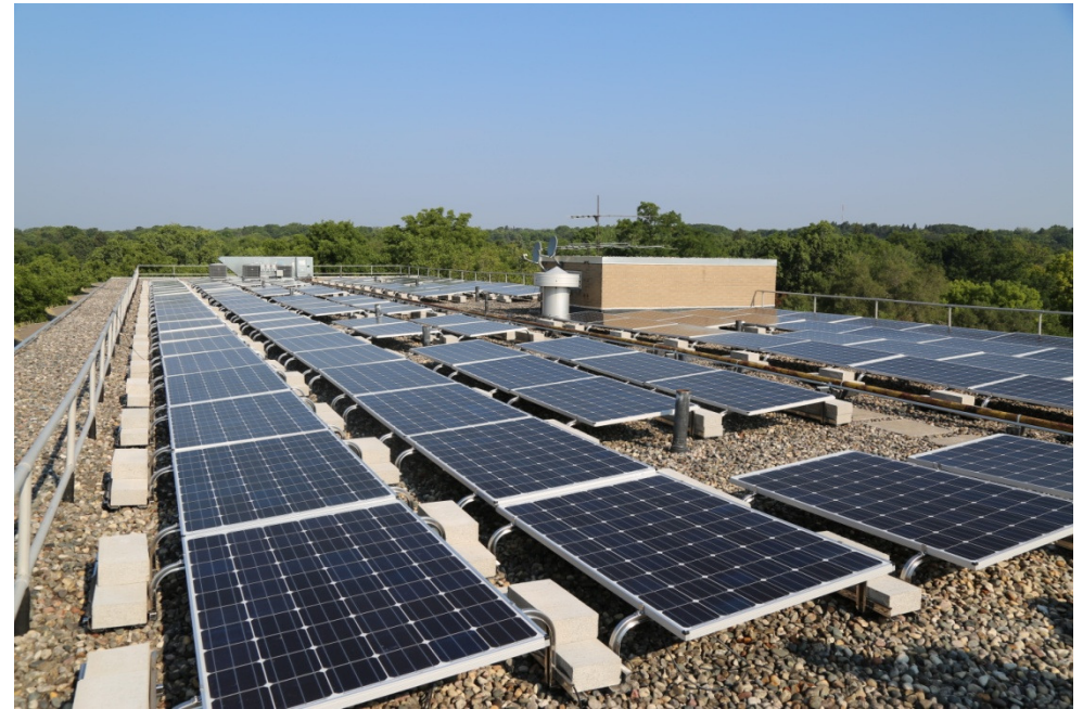
42-kW solar system installed at Miller Manor in 2015
