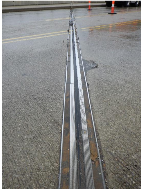
Photograph No. 7 Spalling and Delamination along South Expansion Joint Looking East
