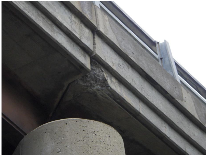
Photograph No. 26 East Deck Fascia Spall at North Pier
