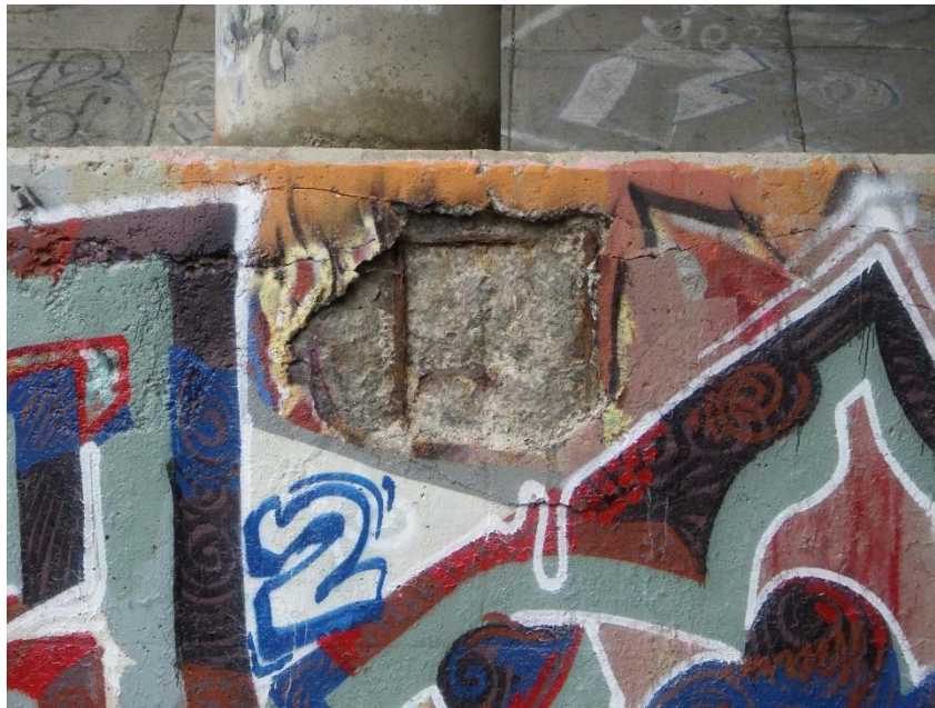
Photograph No. 14 Spalled Crashwall and Exposed Reinforcement on North Side of South Pier under Column 2 (Pier 1)
