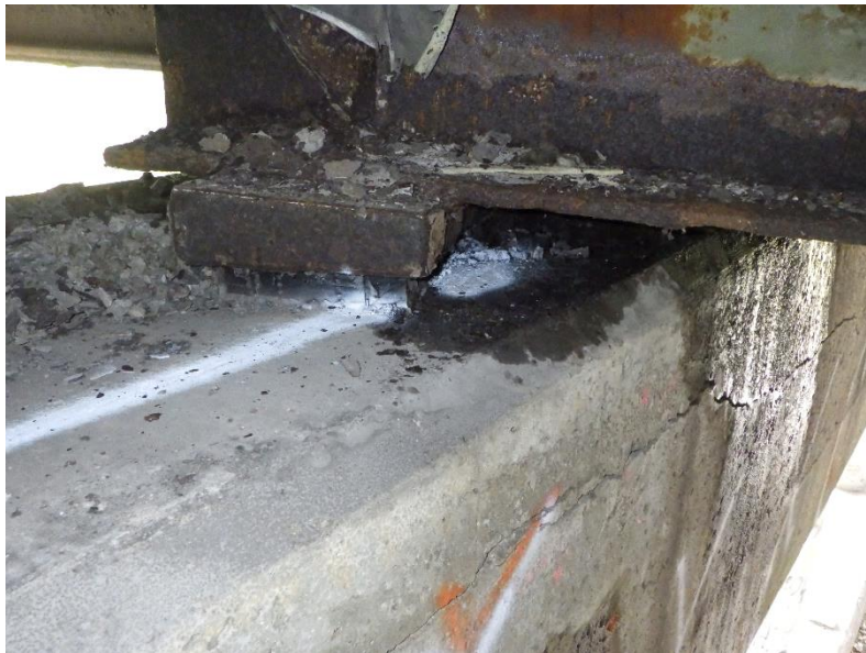
Photograph No. 16 Location of Spall on North Face of North Pier at Edge of Bearing Pad
