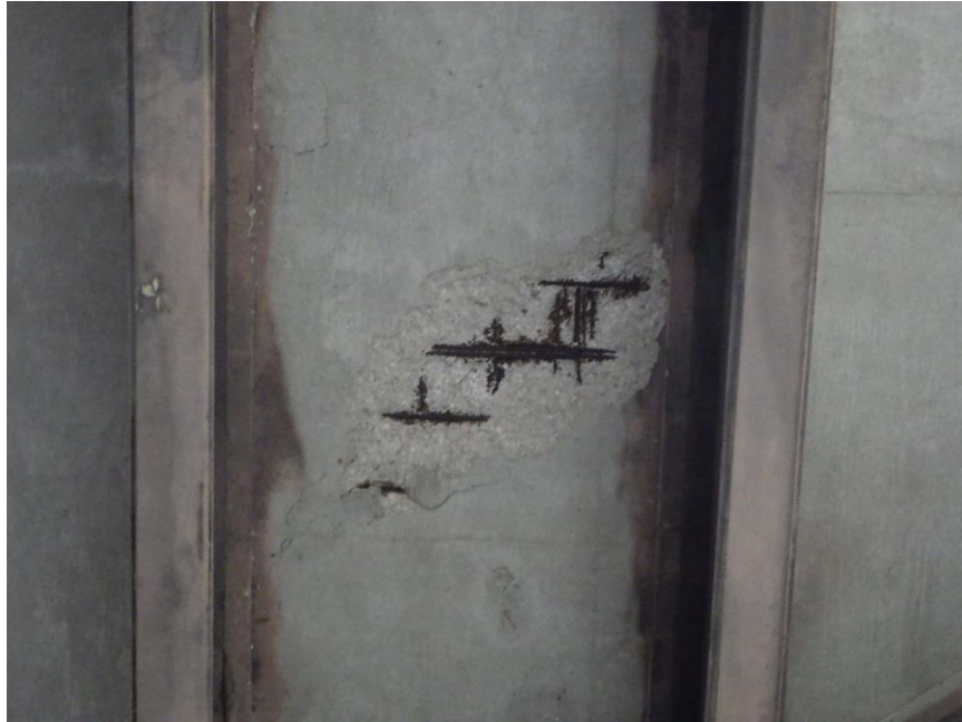
Photograph No. 13 Spalled Concrete with Exposed Deteriorating Reinforcement on Bottom of Deck
