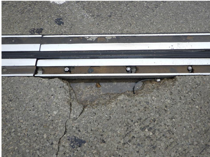
Photograph No. 8 Loose South Expansion Joint
