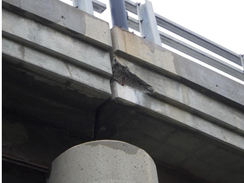
Photograph No. 25 West Sidewalk Fascia Spall at South Pier
