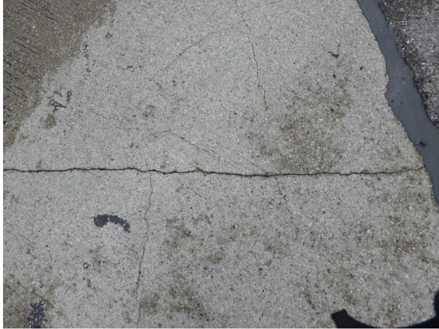
Photograph No. 11 Typical Cracking in Deck
