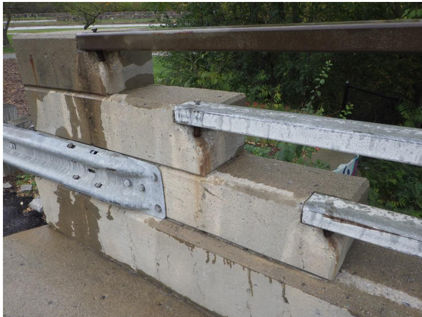
Photograph No. 10 Spalling in Railing End Wall at the Northeast Quadrant
