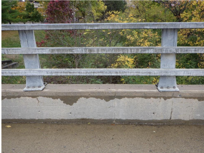
Photograph No. 9 Typical Vertical Cracking in Railing
