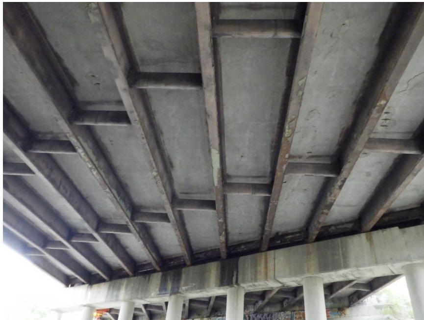
Photograph No. 12 Delaminations on Bottom of Deck with Moisture, Leaching, and Exposed Rebar
