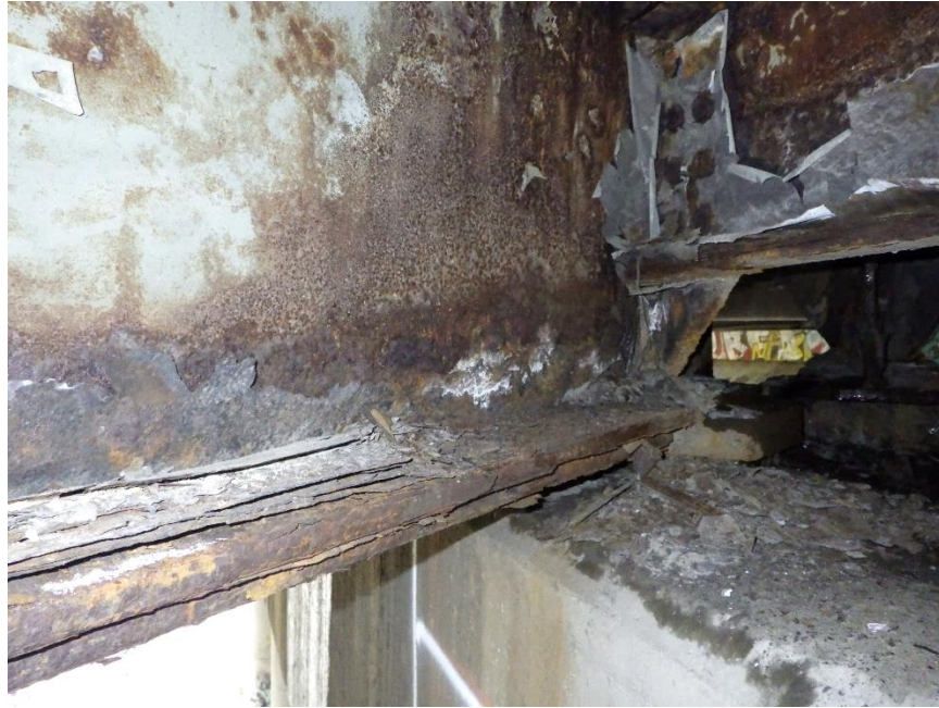
Photograph No. 15 Deteriorated Beam End and Diaphragm at Pier
