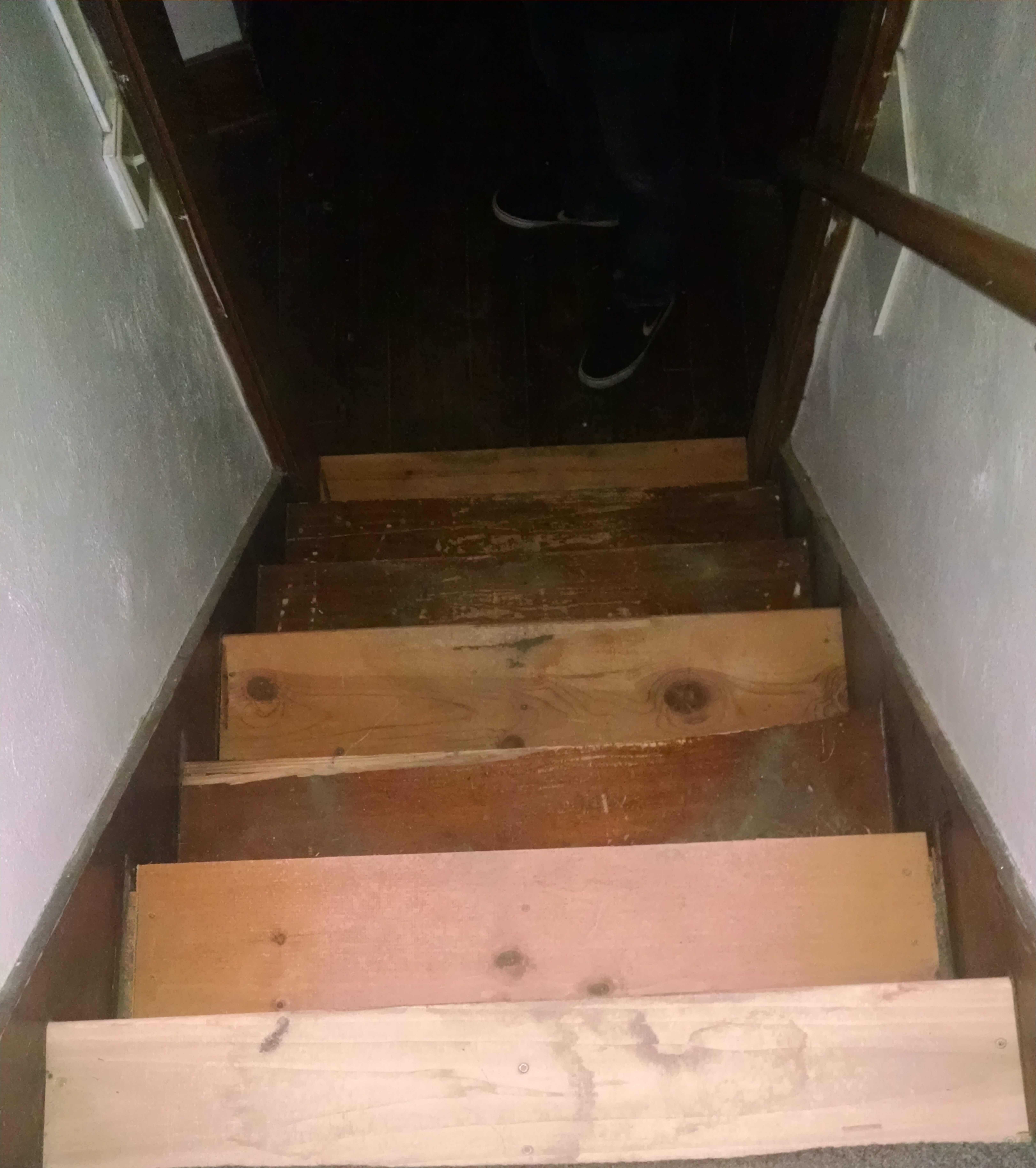
814 SYBIL NONCOMPLIANT STAIR TREADS 2ND FLOOR STAIRWAY
