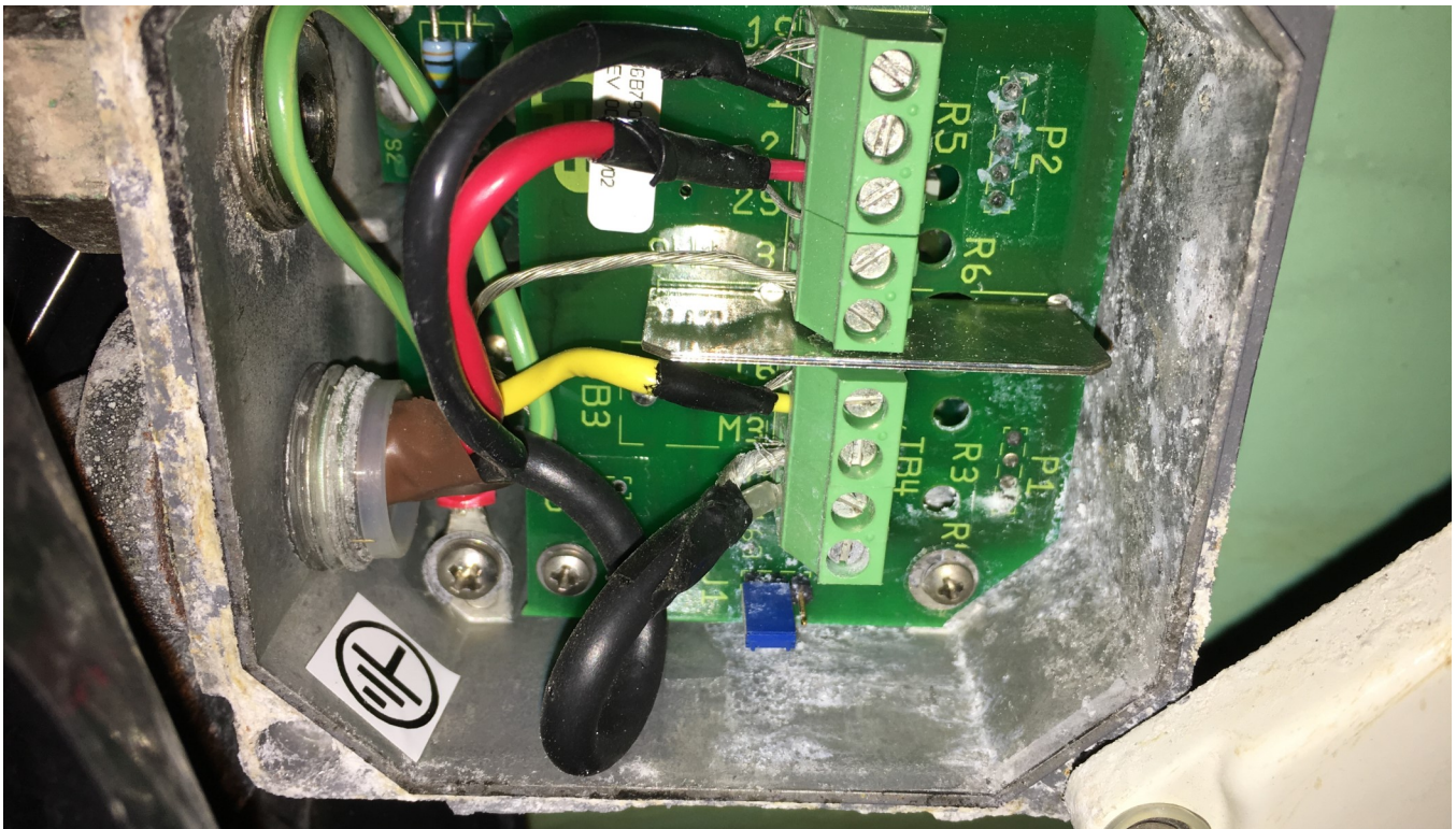
ABB Filter Effluent flow meter. Device not functioning. Typical of 16.
