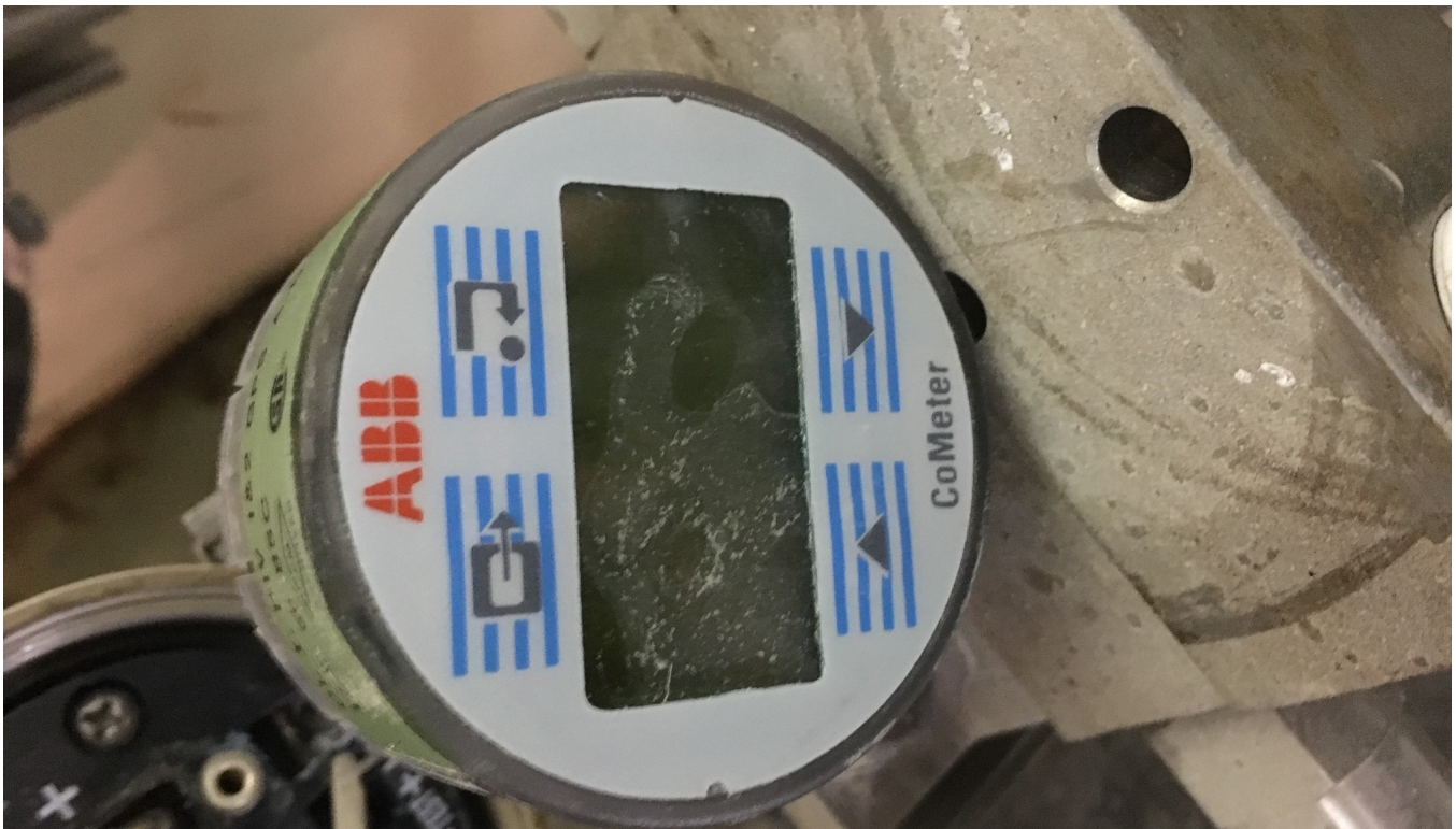
ABB Filter Headloss Sensor Display. Display was immersed and is not functioning. Typical of 16.
