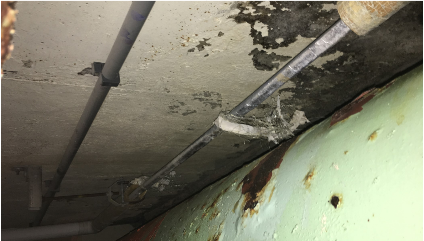
Sodium Hydroxide heat trace and insulation. Line was submerged. New heat trace cable and insulation is needed.
