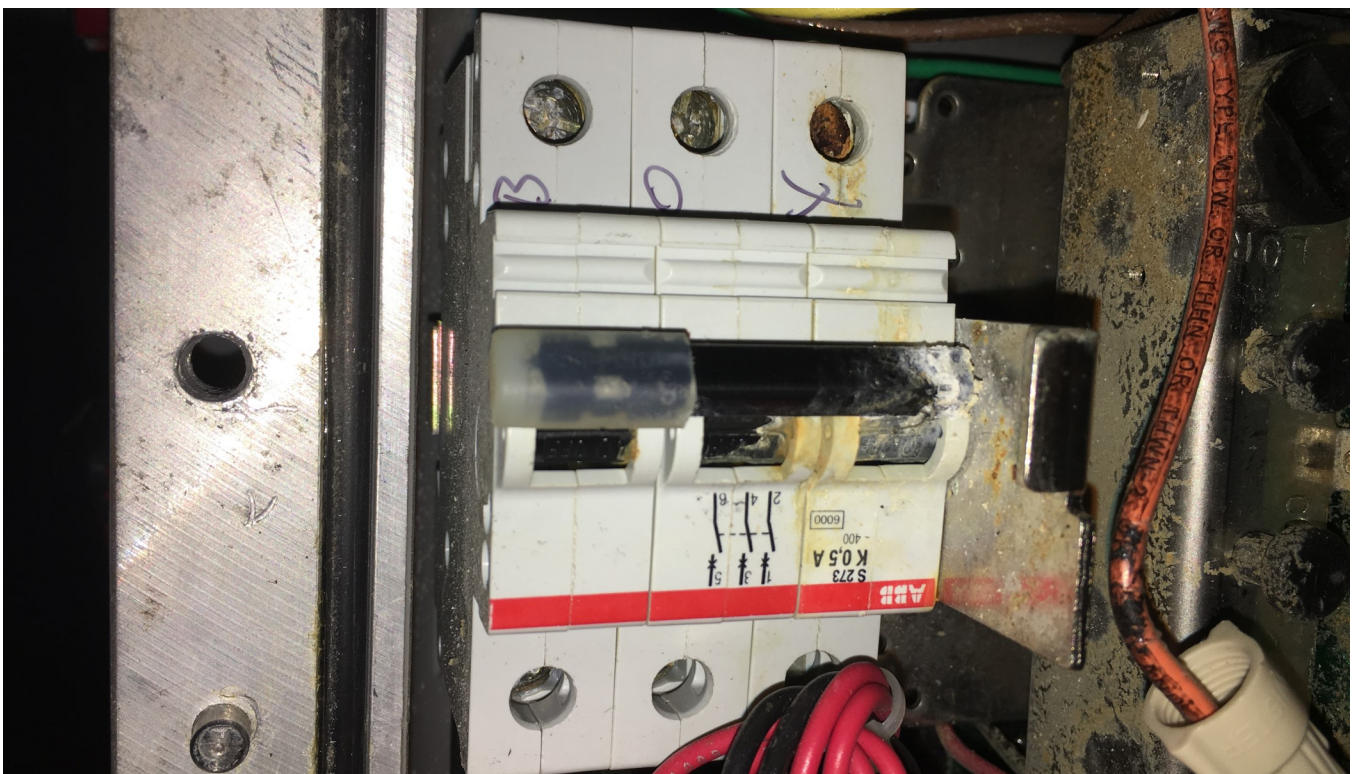
EIM Valve actuator 480V power supply breaker. Breaker was submerged when water entered the enclosure. Wires corroding. Actuator not functioning. Typical of 21.
