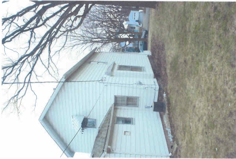
TOP PHOTO OF ORIGINAL 2 STORY HOUSE WITH ADDITION AT LEFT AND PATIO.
