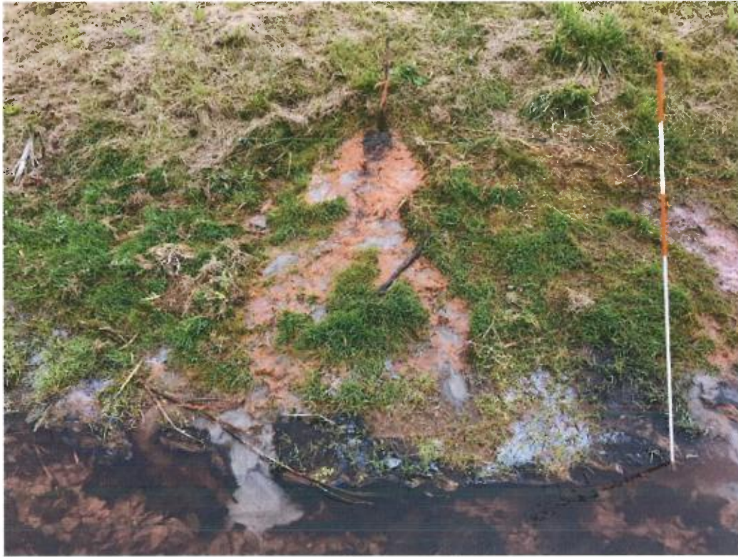
Photo 3: Close up of Boil
