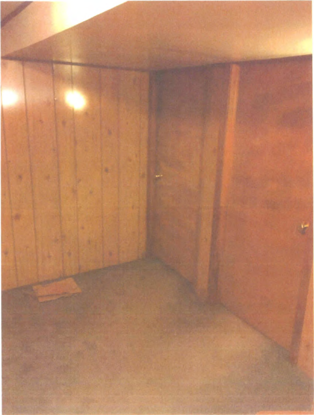
Item 7- Unit 2- 6'4" existing headroom outside of cellar rooms.
