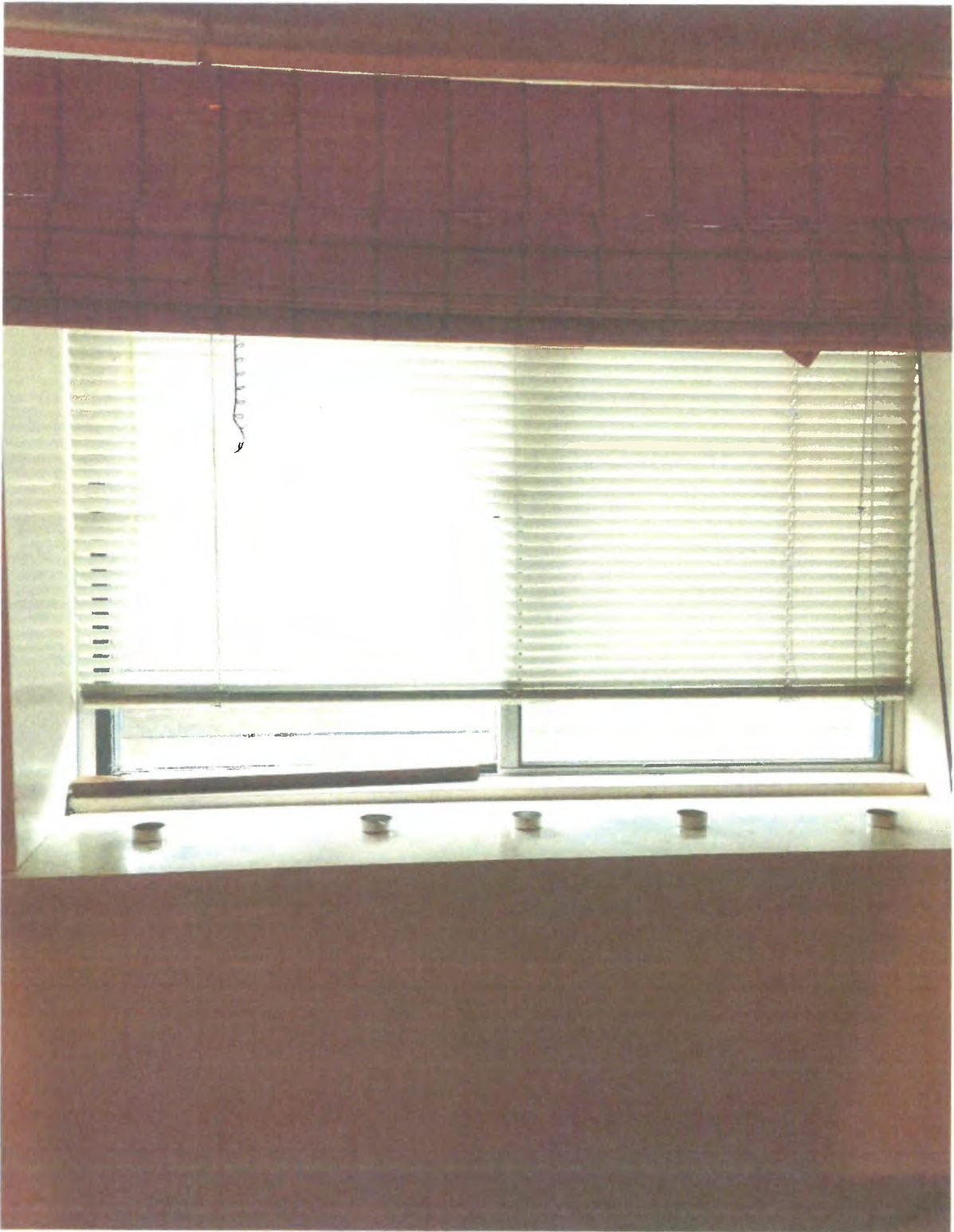
Item 8- Unit 2- Existing slider window in E cellar room for egress with clear opening of 18 \frac{3}{4} " x 30 \frac{1}{2} " and sill height of 50 \frac{1}{2} ".
