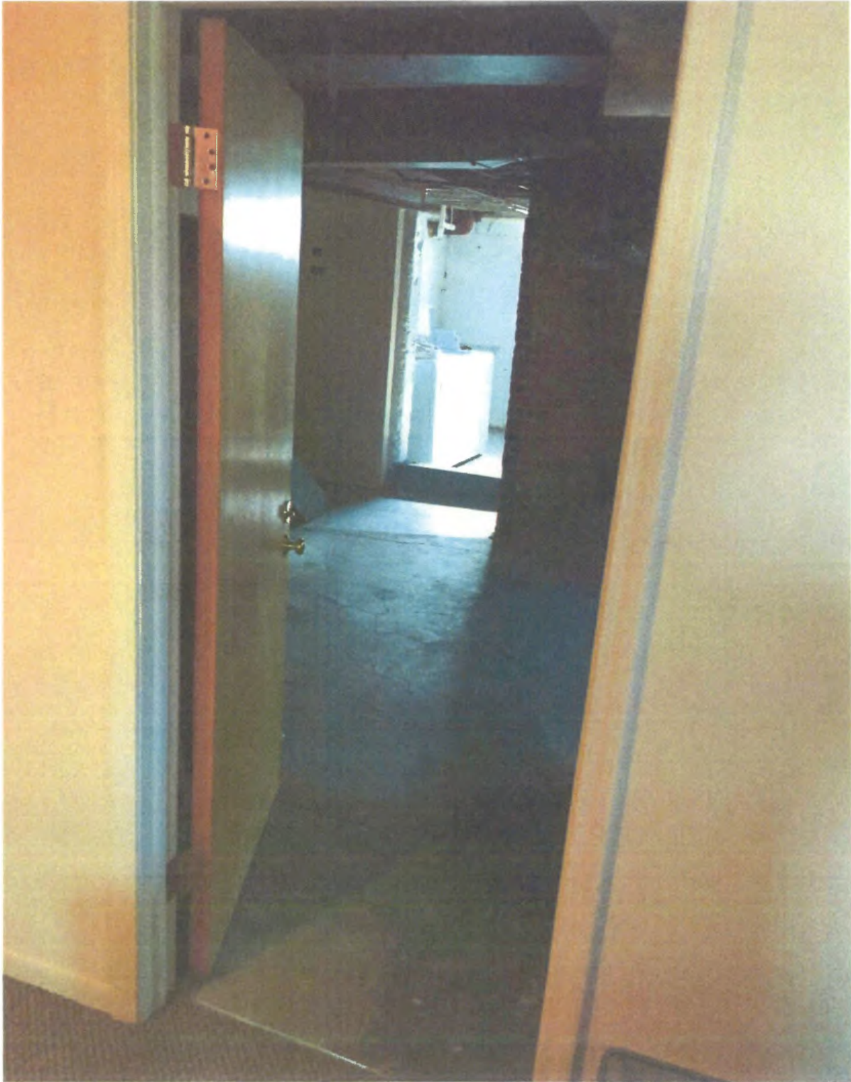
Item 1- Unit 1- Proposed 2nd means of egress from cellar room into mechanical room. 32' self-closing solid core fire door.
