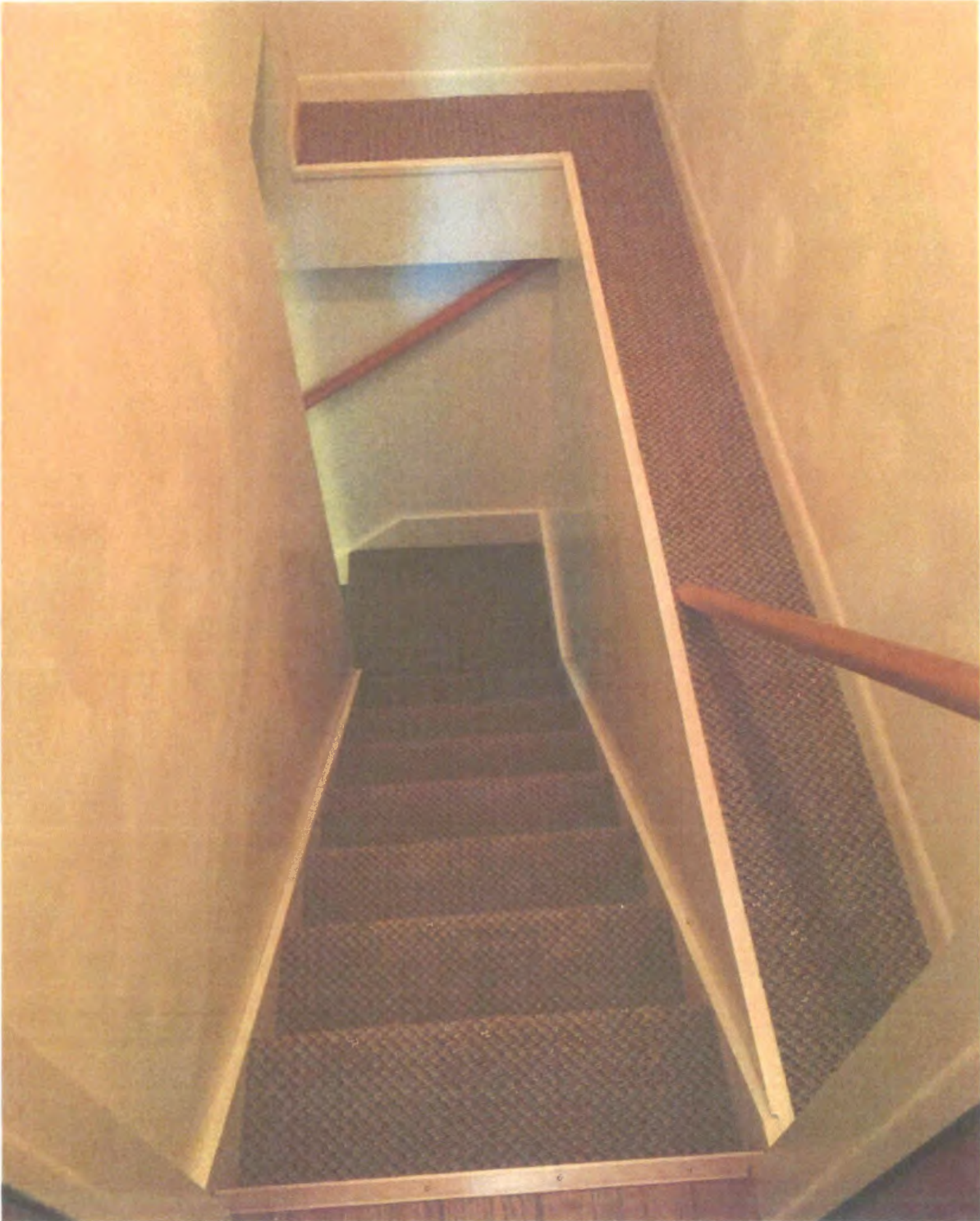
Item 2- Unit 1 cellar stairs. 25" tread-width at bottom of stairs. Wireless, interconnected smoke detectors are at the top and bottom of stairs.
