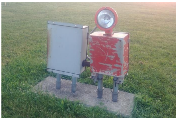
FAA-Owned Runway End Identifier Light
