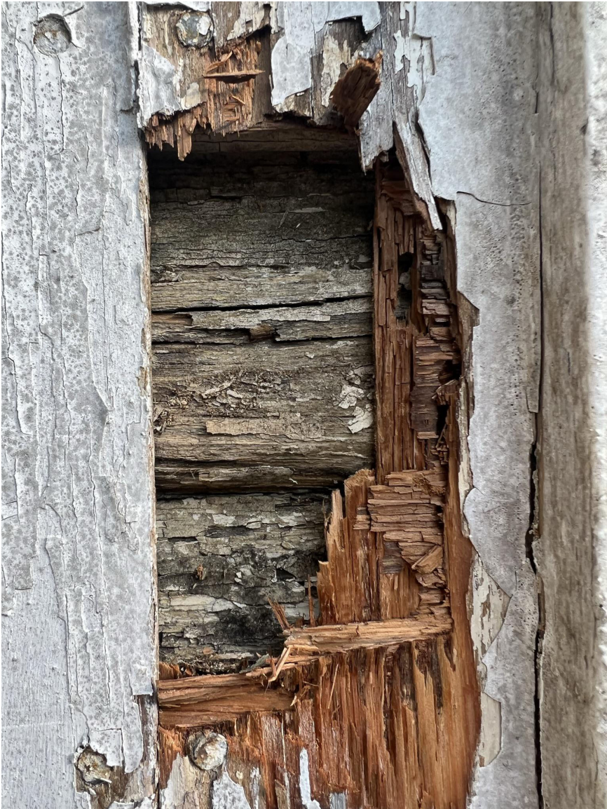
Photo of deteriorated historic cladding behind plywood covering.
