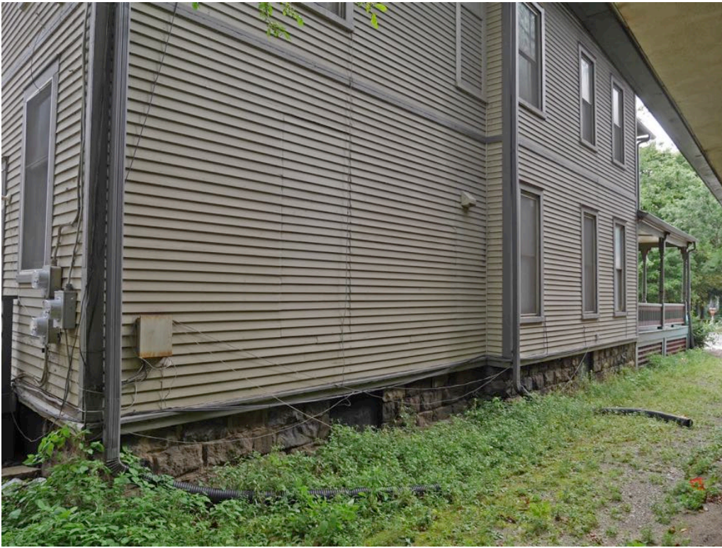
Photo No. 15 (image No. 40): North elevation retains its windows in the western half of the house, but those in the eastern half were blocked up and covered with siding. Mortar joints exhibit eroded and missing mortar.
