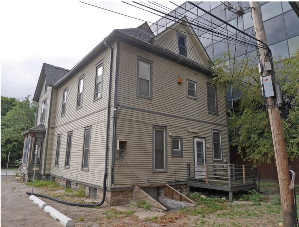
Photo No. 16 (image No. 44): East elevation is where most change has occurred. The original "back" door has been changed to a small window, and a new door added that leads into the modern kitchen. Cellar door cover is missing.
