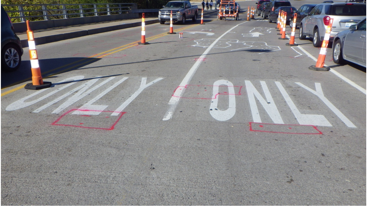
Figure 3 Deck Delaminations in Center Span (looking north)
