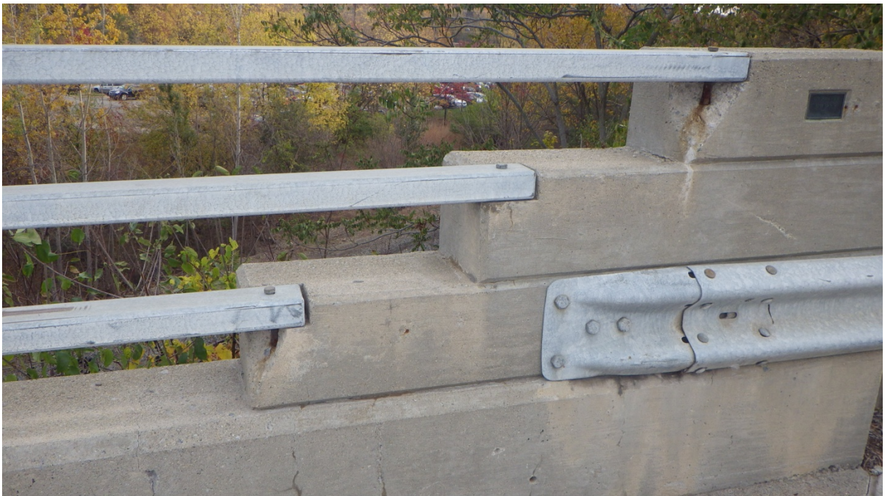
Figure 16 Typical railing end block failures
