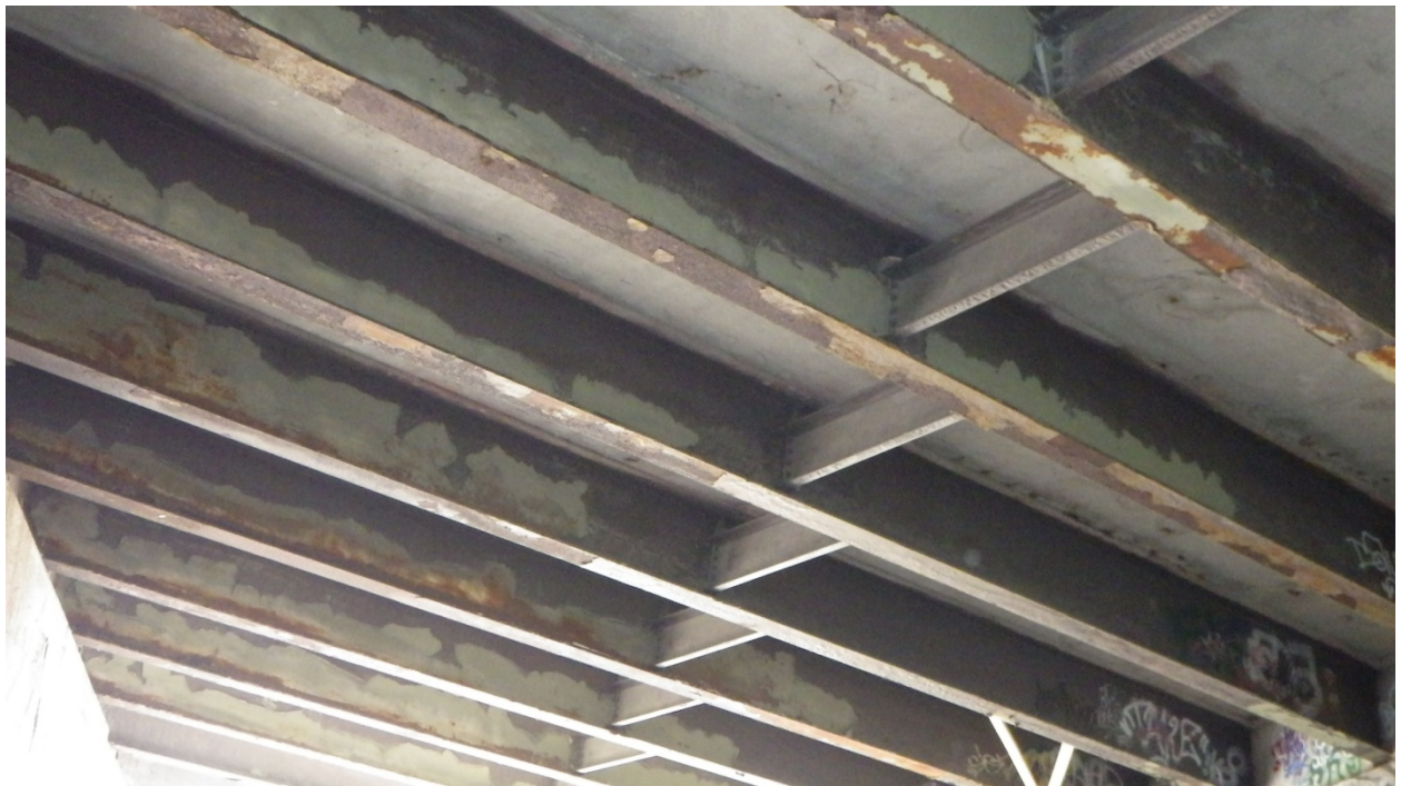
Figure 10 Typical Paint Failure
