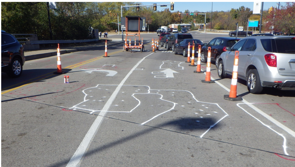
Figure 2 Deck Delaminations in North Span (looking north)
