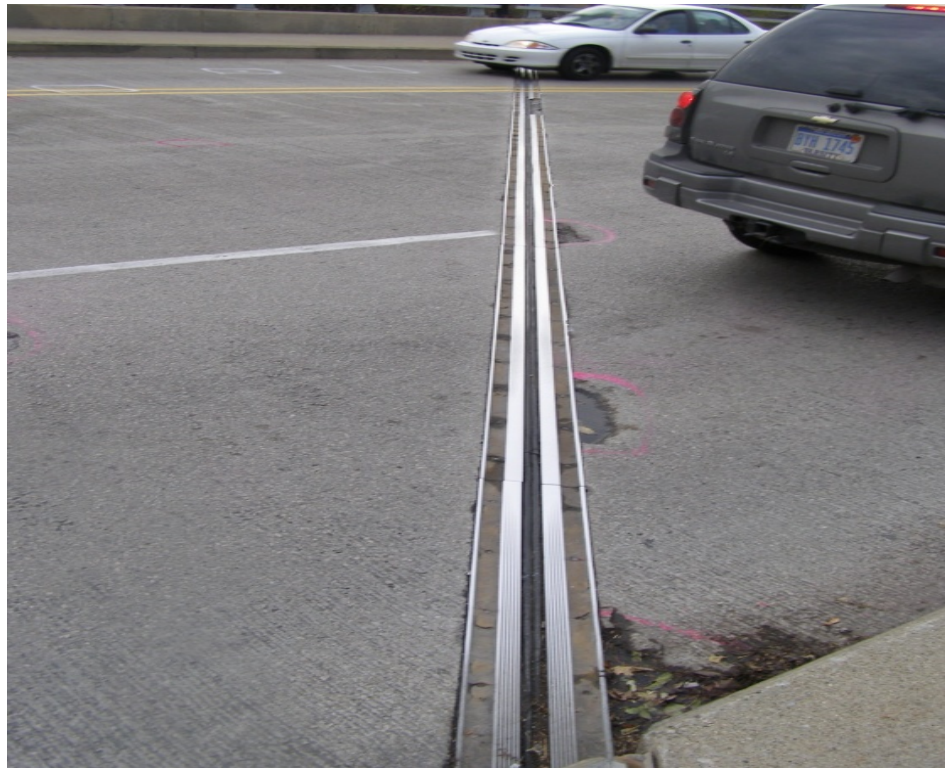
Figure 7 Spalling along South Expansion Joint (looking west)
