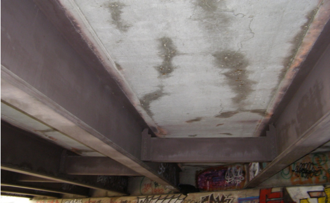
Figure 5 Moisture and Cracking in Bottom of Deck, Span 3
