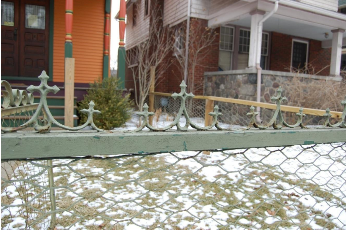
Photograph 13 – Detail of wood and wrought iron fence at 442 South Fourth Avenue, February, 2010
