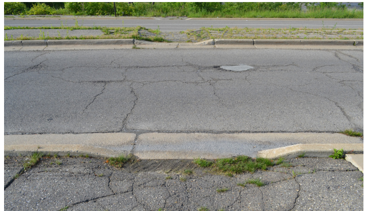
Sidewalks and pedestrian crosswalks are deteriorated
