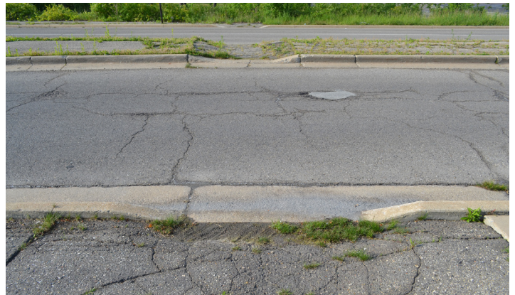
Sidewalks and pedestrian crosswalks are deteriorated
