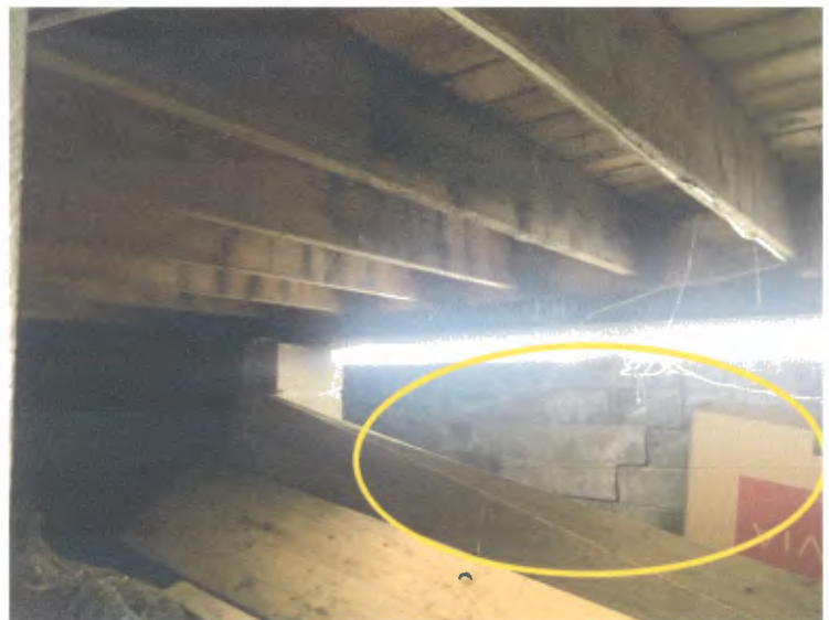
Failing foundation underneath garage
