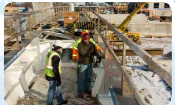
The cold prohibits some types of work at the site, but the project moves ahead despite the weather.
