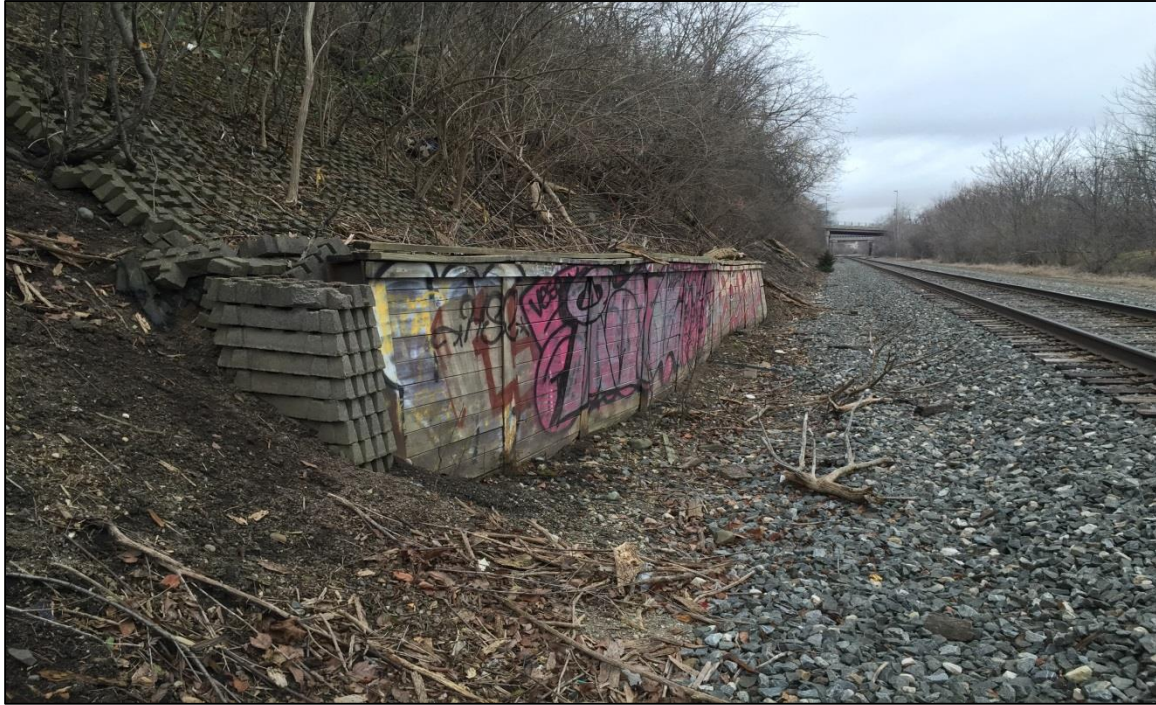
PHOTO NO. 9: Looking west at the soldier pile retaining wall at the toe of the slope.
