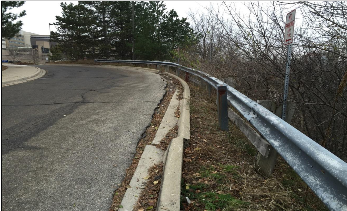
PHOTO NO. 1B – December 12, 2015: Looking west along the north curb line of Nichols Drive. Inclinometer I-2 is also visible in this photo between the guardrail and the curb line.
