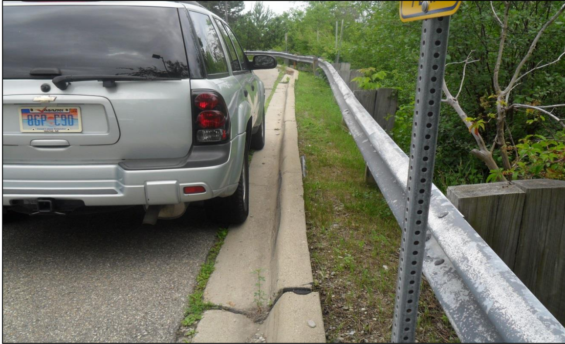
PHOTO NO. 3A – June 11, 2010: Looking west along the north curb line of Nichols Drive.
