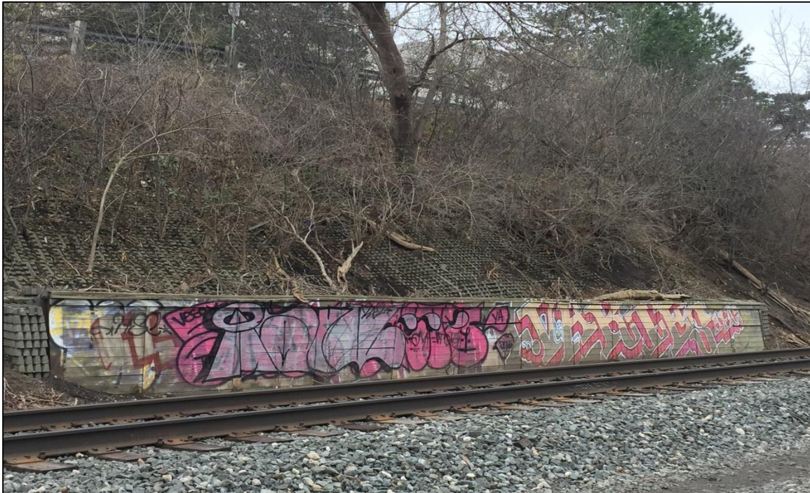
PHOTO NO. 4B – December 12, 2015: Looking at the soldier pile retaining wall from a similar vantage point as PHOTO NO. 4A.
