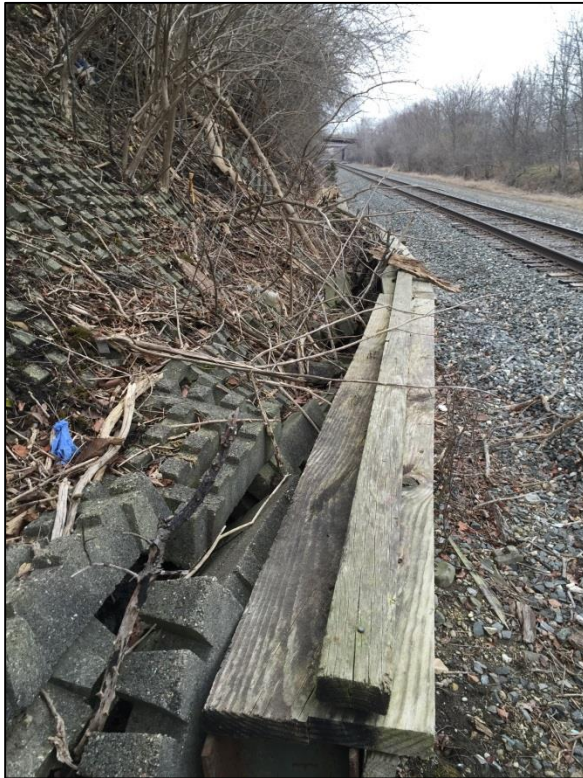
PHOTO NO. 10: Looking west along the top of the soldier pile retaining wall at the toe of the slope.
