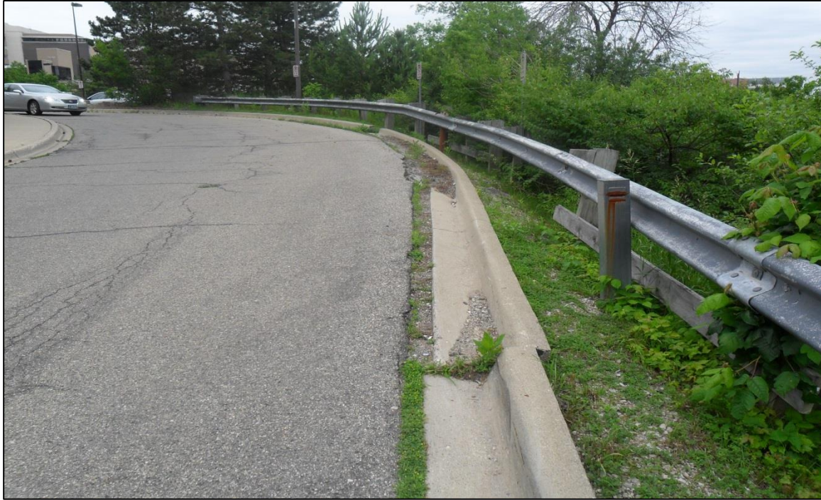
PHOTO NO. 1A –June 11, 2010: Looking west along the north curb line of Nichols Drive. Inclinometer I-2 is in the right of the photo between the curb and the guardrail.
