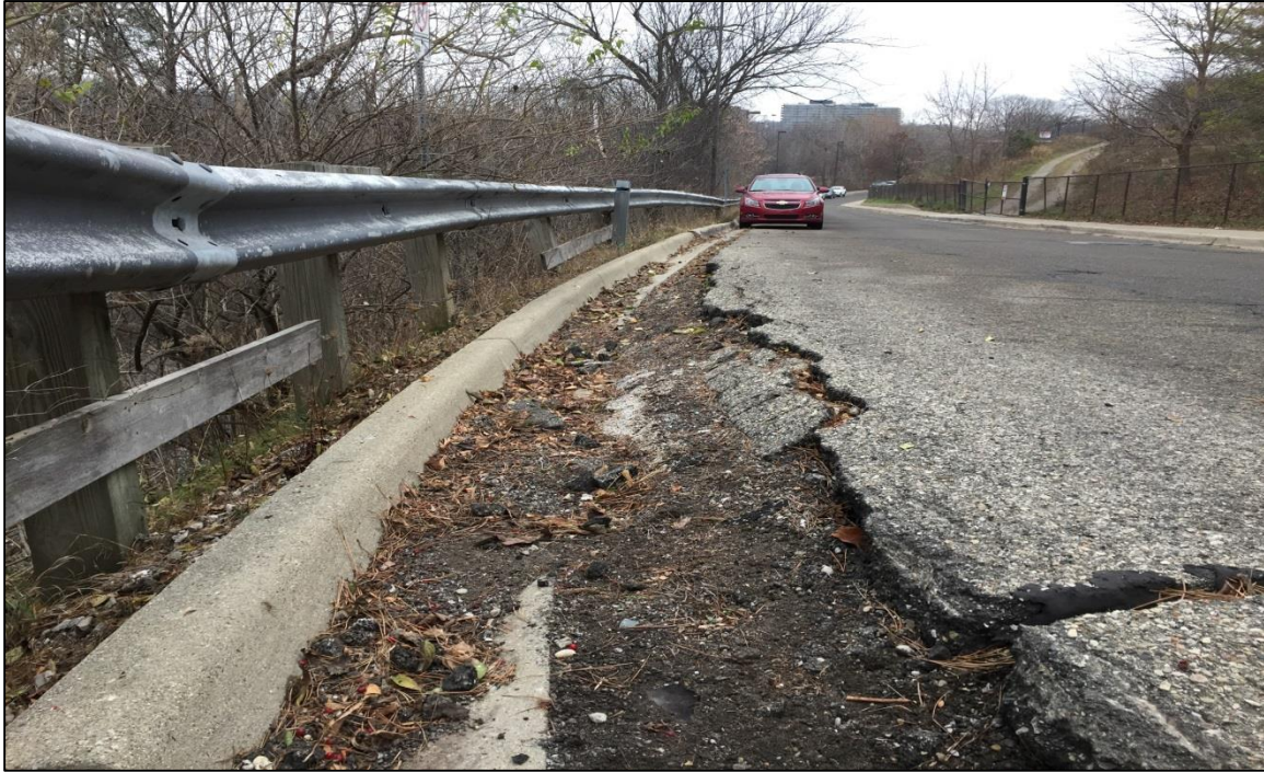
PHOTO NO. 7: Close-up of the drop in the pavement surface along the north curb line of Nichols Drive. Inclinometer I-1 is located immediately to the left of this location.
