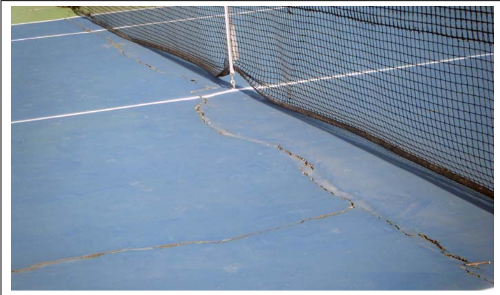
and more Cracks
