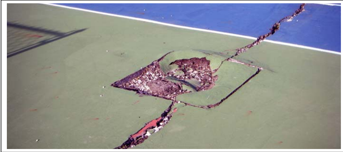
West Court, missing post
