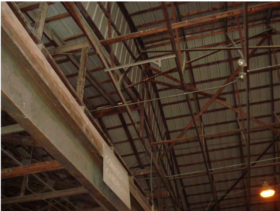
8. Loose bracing and stressed members at the west gable end.
