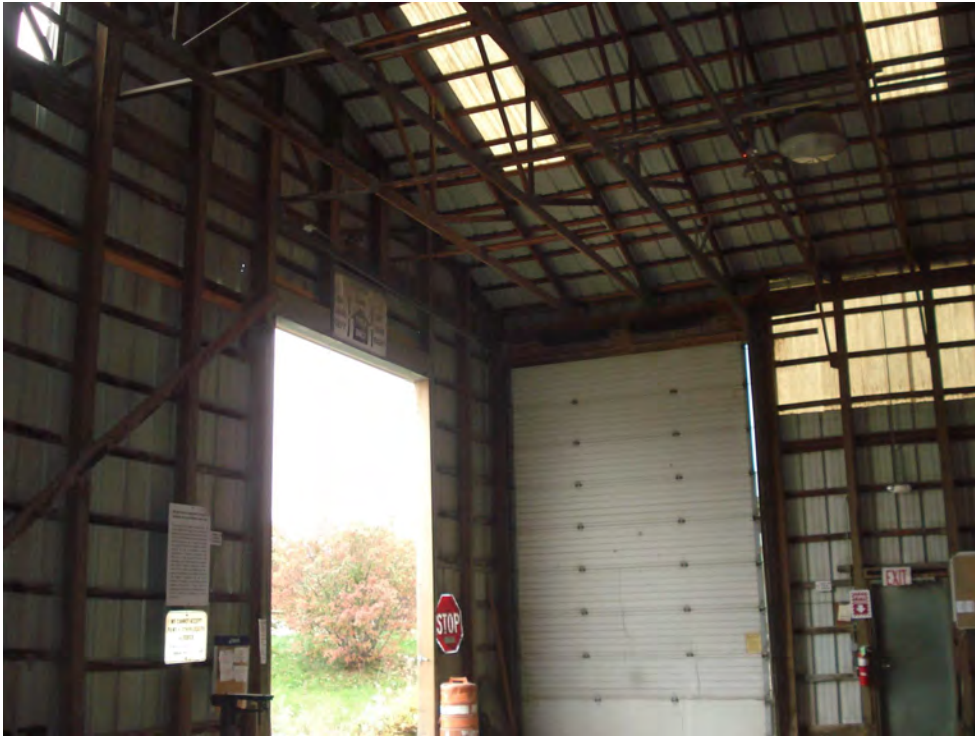
5. Southeast corner of the building has settled at least 12 inches.
