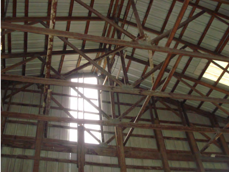
7. Siding gaps and truss movement at the east gable end of the roof.
