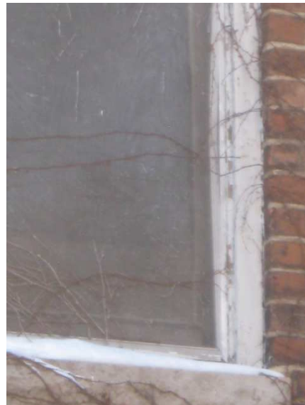
All windows show similar deterioration
