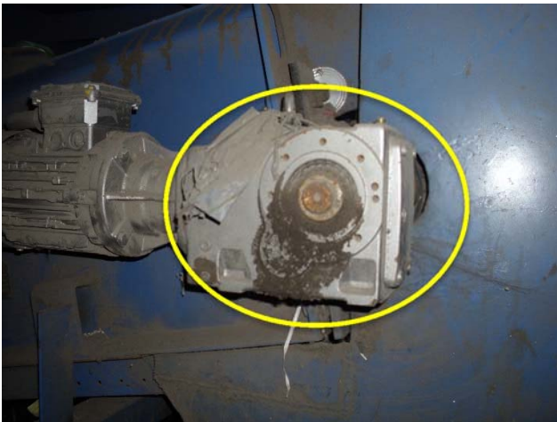
Gearmotor is leaking. It is held stable by zip ties. Replacement required.
