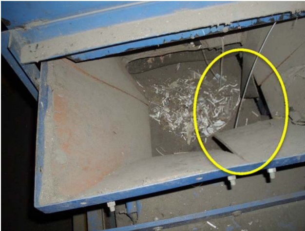
Liners need to be replaced.
