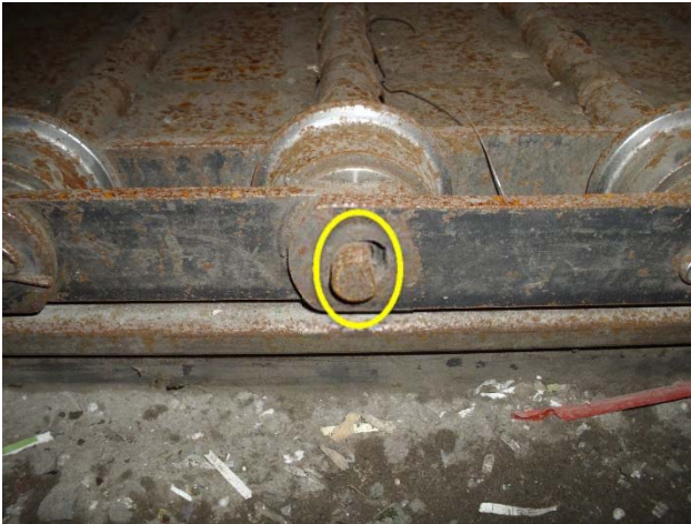
D hole bars are worn out, no cotter pin installed.
