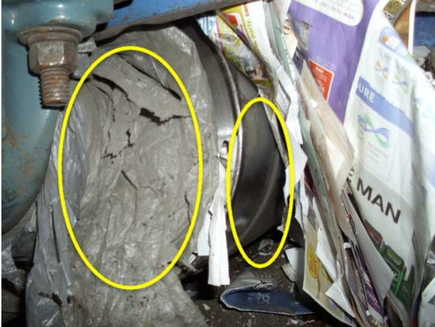
Shaft is wrapped, belt tracking needs to be corrected.
