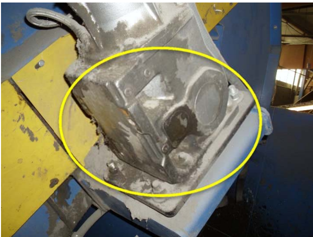
Gearmotors are leaking, replacement required.
