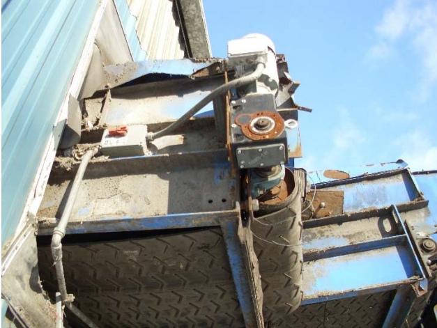
Wire wrapped around pulley and shaft.
