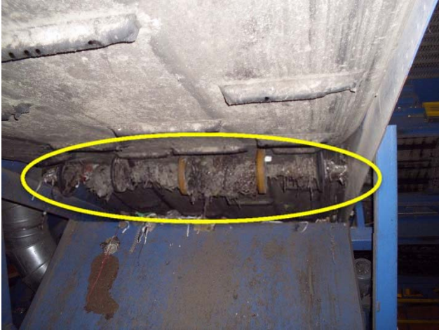
Return rollers are worn and some are omitted. Replacement required.
