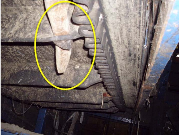
Belt is worn and objects are protruding through cleats, replacement required.
