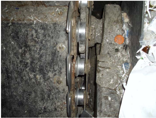
Belt is worn, immediate replacement required.
