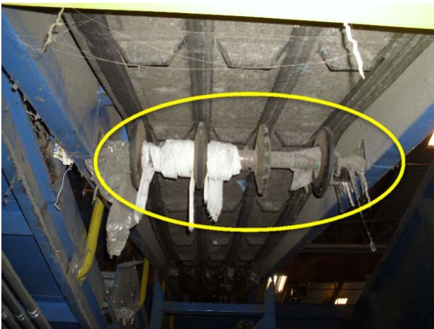
Return rollers are worn and wrapped. Replacement required.
