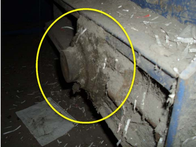
Both head and tail pulley and bearings are severely worn, replacement required.
