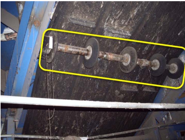
Return rollers are showing signs of wear, but are still serviceable.
