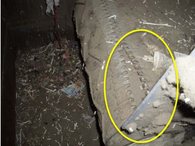
Belt is torn, lacing is ripped, replacement required.
