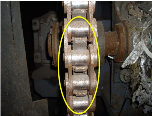
Head sprocket and Motor sprocket needs to be replaced. When sprockets are replaced, it is advised to change chain.
