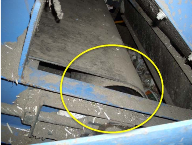
Belt tracking needs to be corrected.
