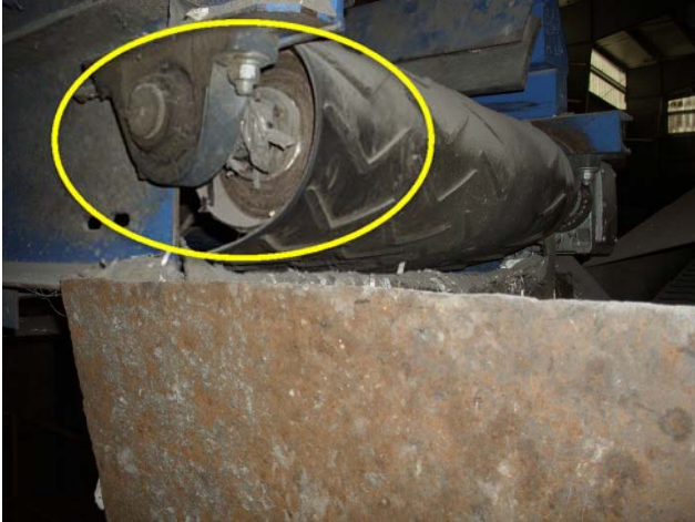
Pulleys and bearings are damaged, replacement required.
