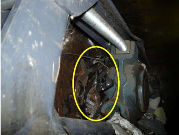
Picture shows wrapped shafts. Take up frame is bent.
