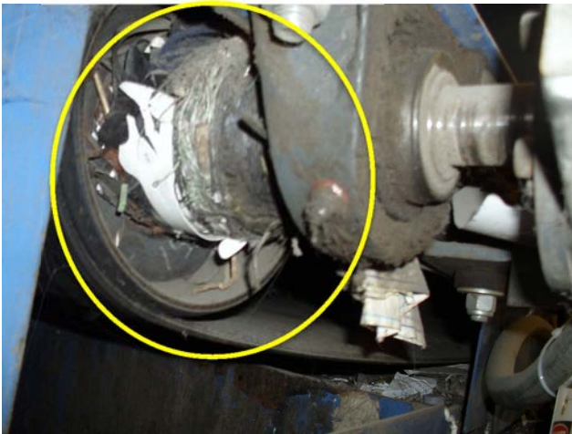
Pulley shafts are wrapped, bearings are worn, replacement of all required.
