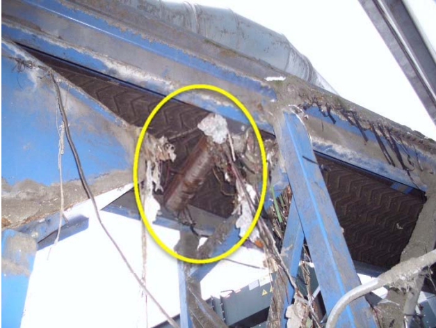
Return rollers are worn, replacement required.
