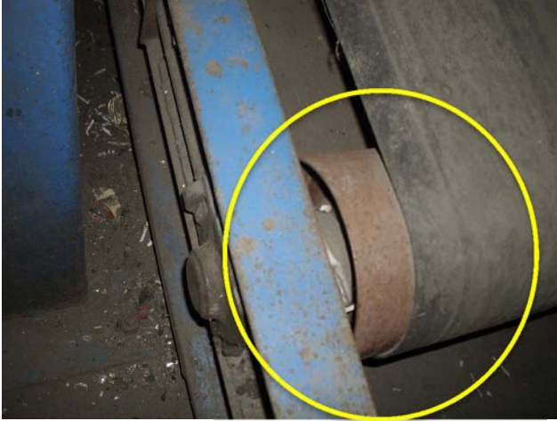
Tracking is to the right, belt is worn.
