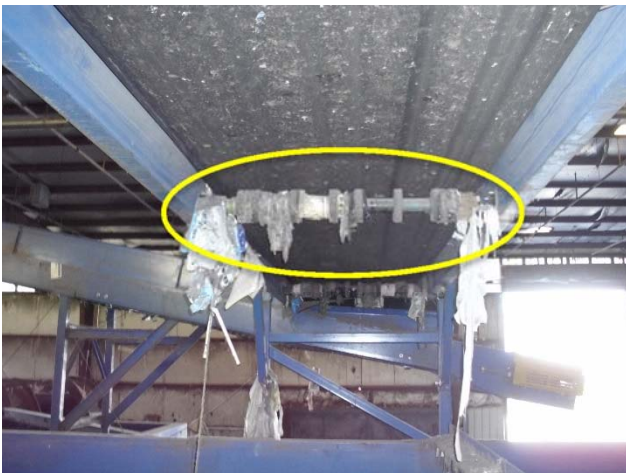
Return rollers are worn and need replacement.
