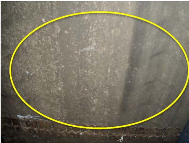
Belt is severely worn, replacement required.
