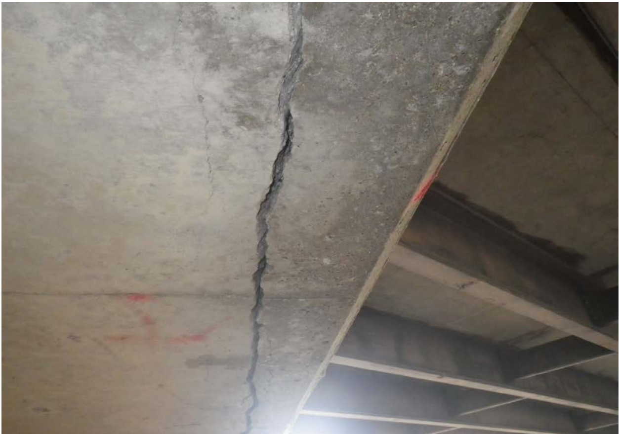
Figure 12 Cracked Pier Cap (North Pier (Pier 2))
