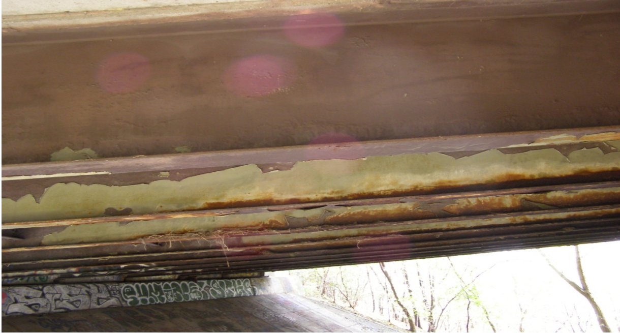
Figure 11 Paint Failures at bottom flange of beams
