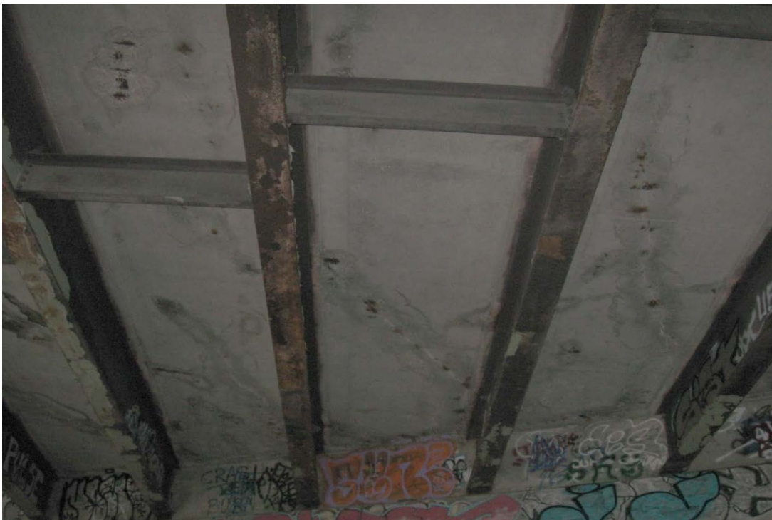
Figure 6 Full Depth Cracks with Moisture, Leaching, and Rust Stains
