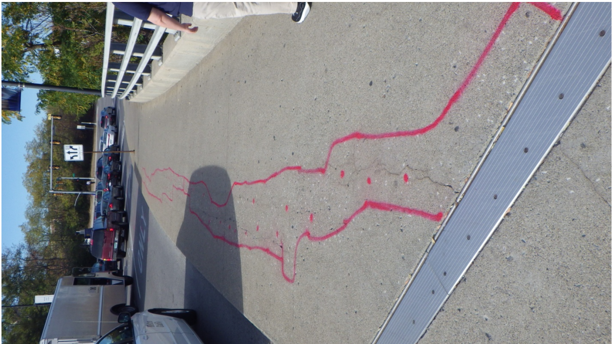
Figure 4 Sidewalk Delaminations on east sidewalk
