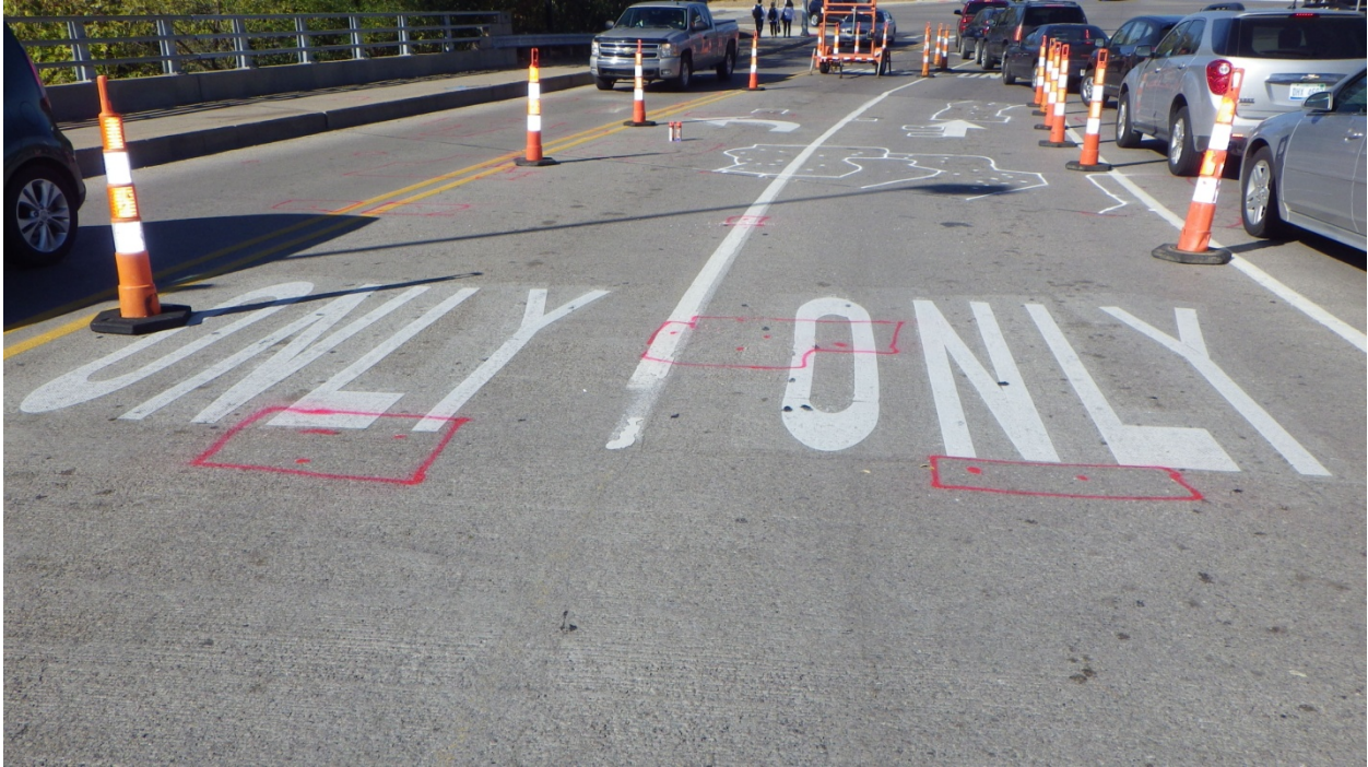
Figure 3 Deck Delaminations in Center Span (looking north)
