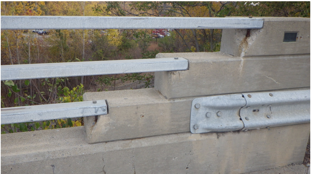
Figure 16 Typical railing end block failures
