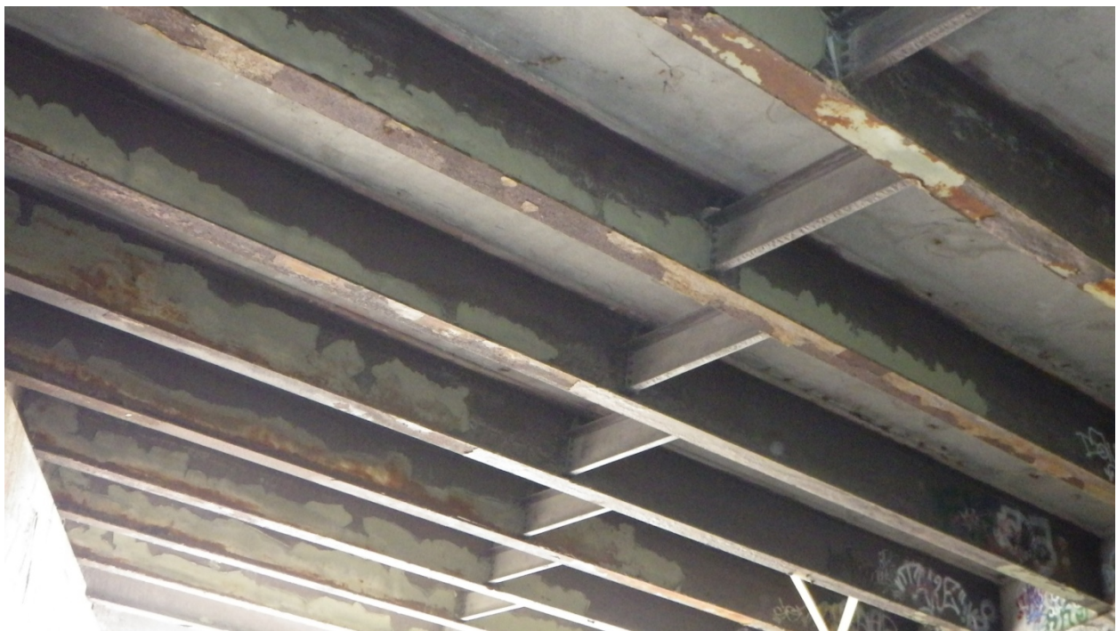
Figure 10 Typical Paint Failure
