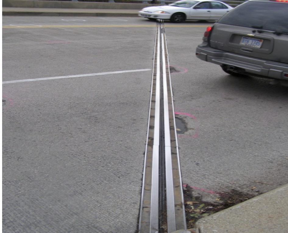
Figure 7 Spalling along South Expansion Joint (looking west)
