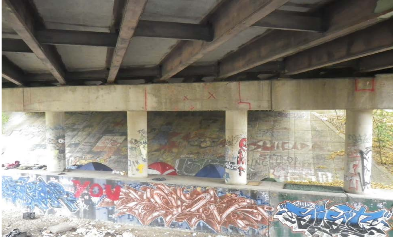
Figure 13 Delamination on South Side of South Pier (Pier 1)
