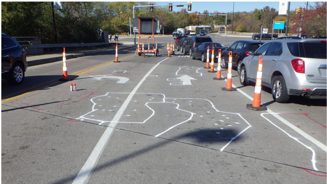
Figure 2 Deck Delaminations in North Span (looking north)
