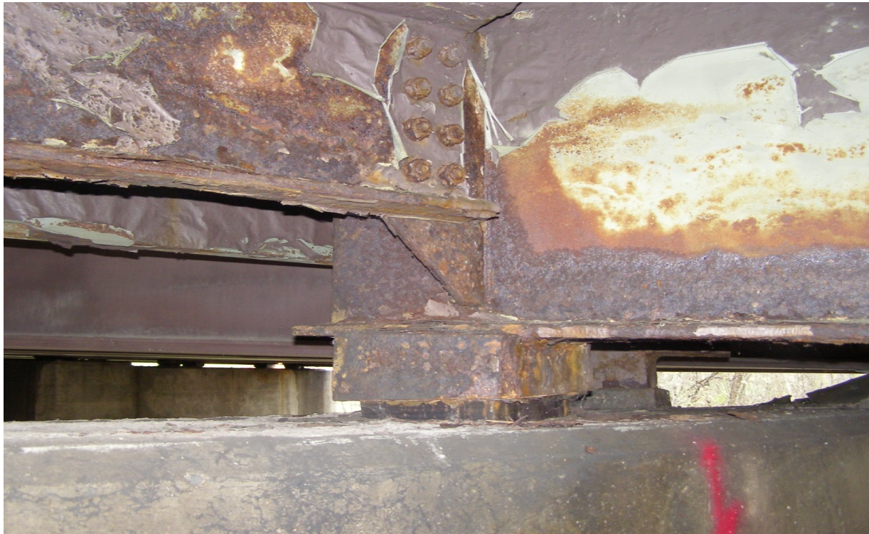
Figure 9 End Diaphragm and Beam End Surface Rusting and Paint Failure, Pier 2
