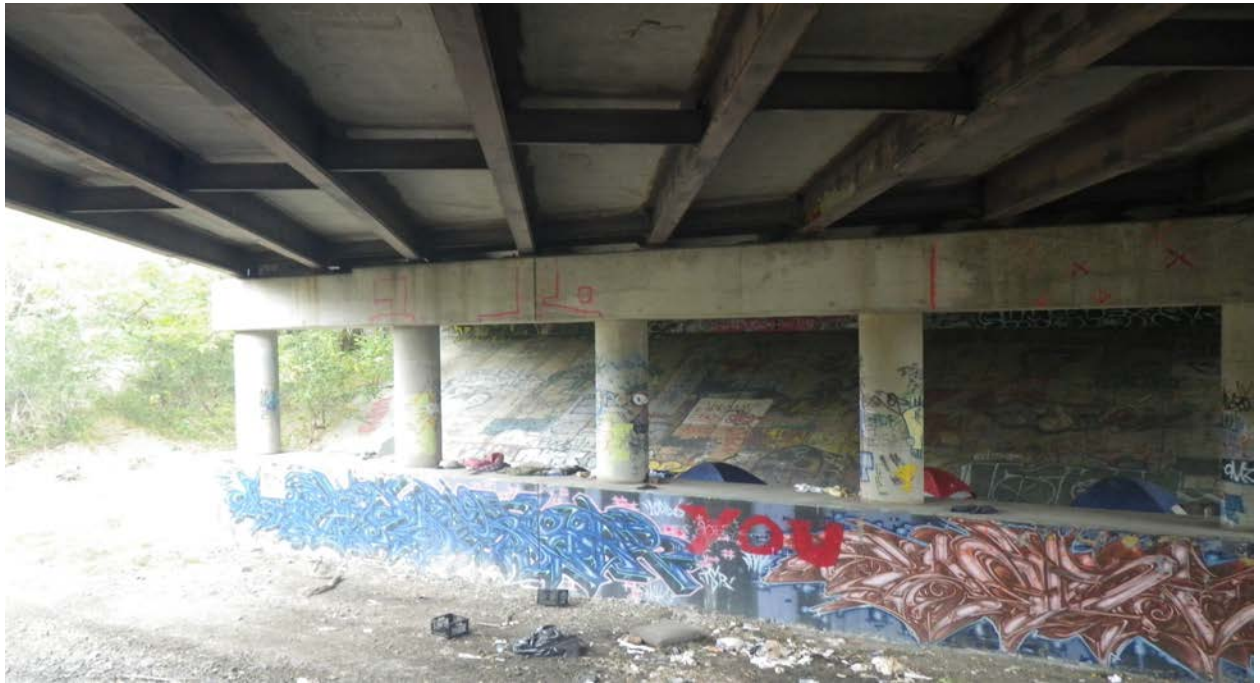
Figure 14 Delaminations on South Side of North Pier (Pier 2)
