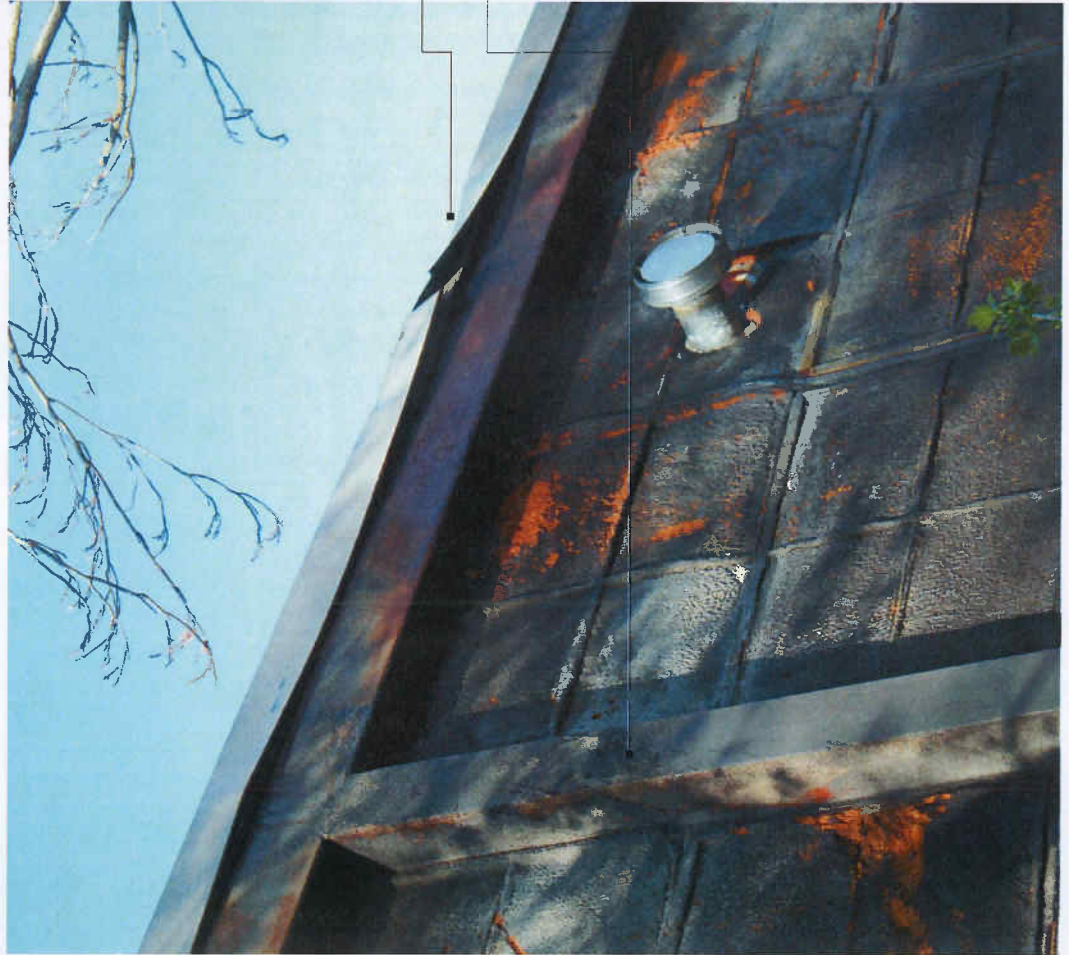
N2.3 Flashing at roof line is separated.
