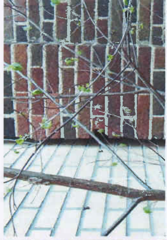
N1.4 The 1 1/2" wide expansion joint between Building 1 & Building 2 appears to be in fair condition. Set back 8" is a copper waterstop which is grouted in place along the continual length of the opening. Some deterioration of the existing brick at Building 1 was observed, as sections of the corner condition have crumbled and broken.
