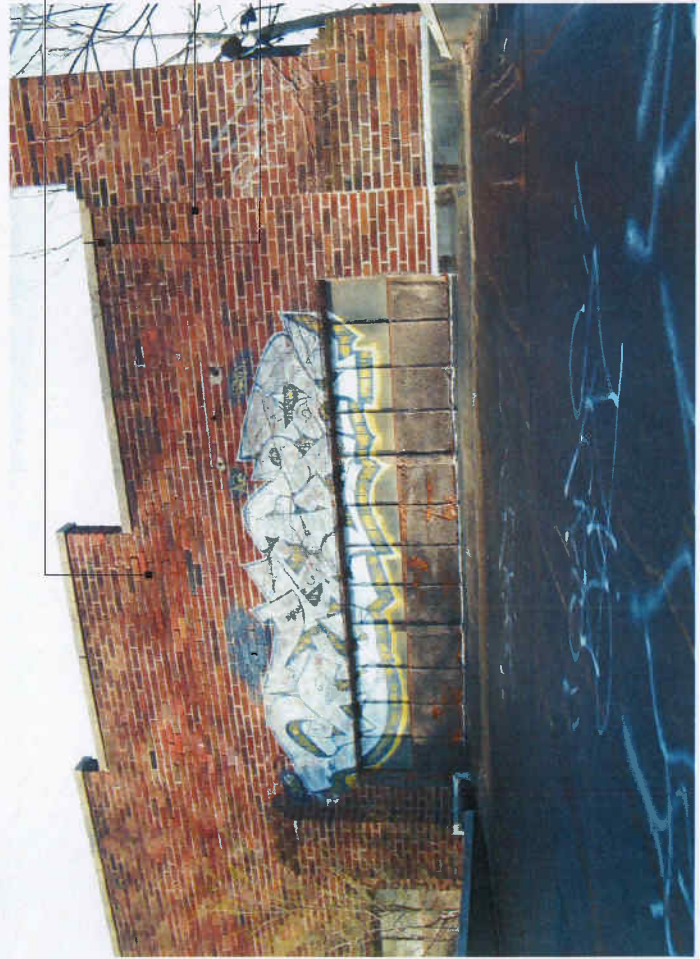
N1.3 The existing brick along the end of the parapet at the approximate location of the vaulted roof line is in poor condition. The mortar has completely deteriorated and sections of brick appear very loose and disconnected from the system. Root cause is likely water infiltration at the flashed joint between the parapet wall and roof.
