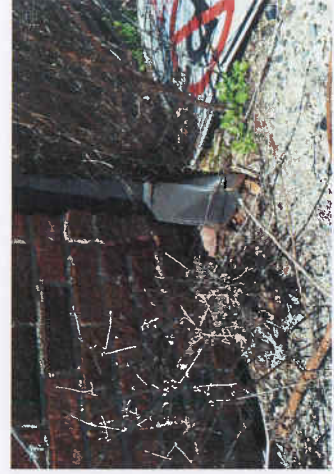
E1.7 Three of the four existing downspouts tie into conductors as part of the existing storm drainage system for the building. A single downspout at the SE corner of the building is disconnected and damaged and currently discharges onto the adjacent concrete paving. Overall the downspouts and conductors appear to be in fair condition with evidence of semi-recent maintenance.
