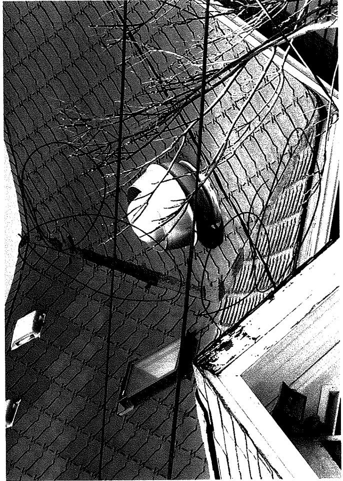
DETERIORATED SHINGLES + VALLEYS VALLEY REPAIR SHOWN
