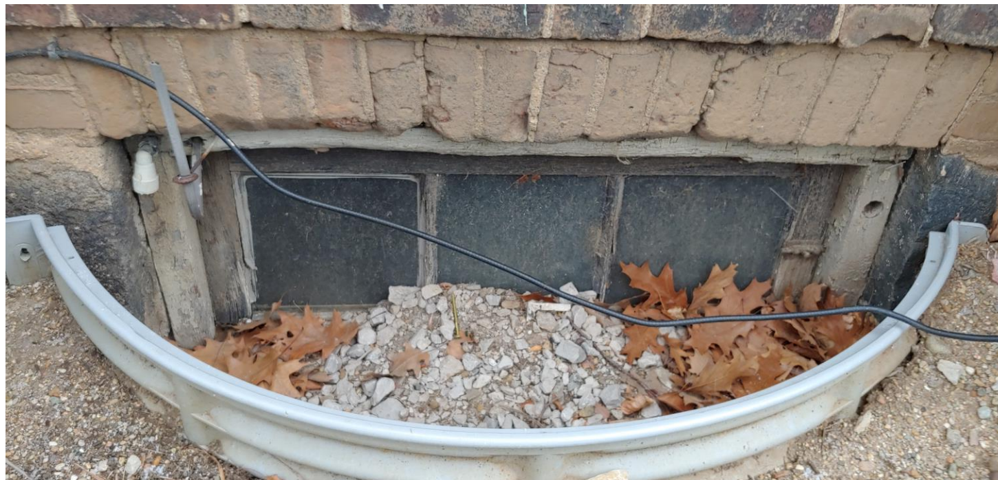
Existing 3 lite wood window approx. 34" W x 16" H with 2" wood trim around it It is 6" from top of window to grade
