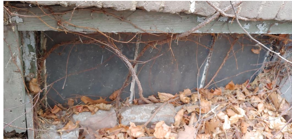
Existing 3 lite steel window approx. 34" W x 16" H with 2" wood trim around it It is 6" from top of window to grade
