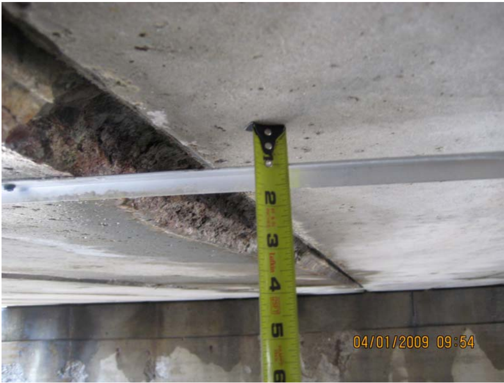
The Failing Beam at the Stadium Bridge over State Street
