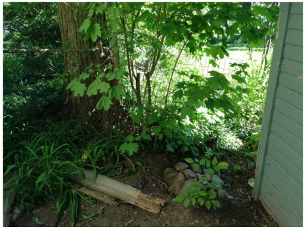
Other side of rear lot line where a small stretch of wire fencing needs to be replaced with new wire fencing.
