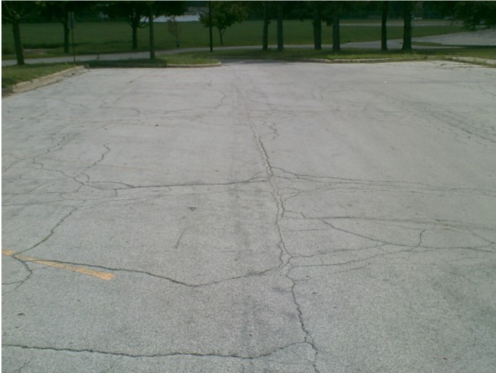
Photograph No. 3: Moderate severity longitudinal and fatigue cracking in north parking lot.
