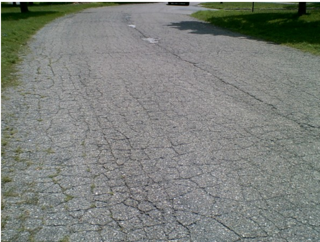
Photograph No. 4: High severity fatigue cracking in north access drive. Note previous patching.
