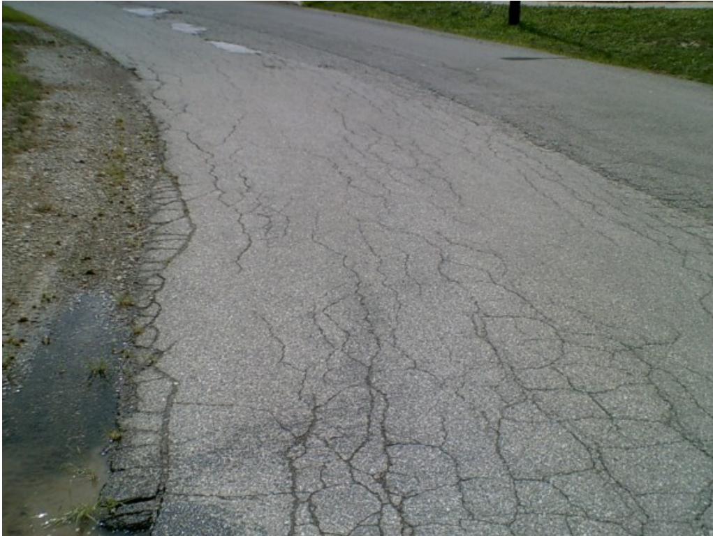
Photograph No. 15: High severity fatigue cracking and edge deterioration (with ponding water) in access drive.
