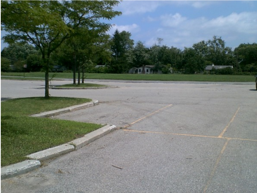
Photograph No. 13: View of overall south parking lot. Pavement is in moderate condition.
