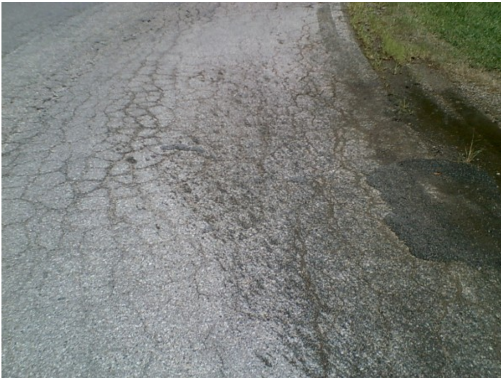
Photograph No. 14: High severity fatigue cracking in access drive.
