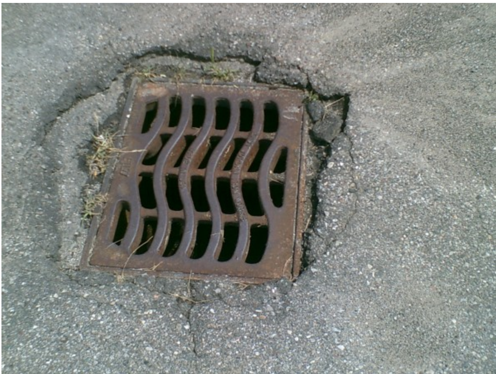
Photograph No. 12: Settlement and deterioration of bituminous pavement around catch basin.
