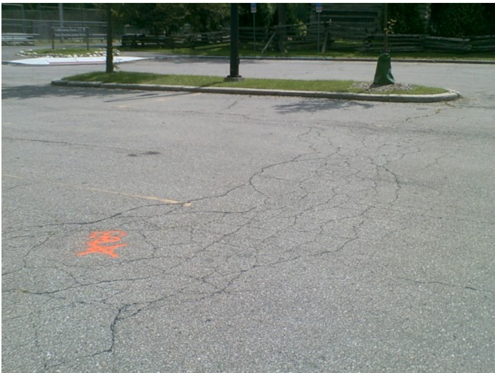
Photograph No. 8: Moderate severity fatigue cracking in south parking lot.
