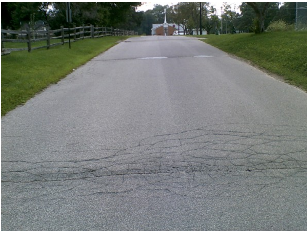
Photograph No. 18: Areas of moderate severity transverse and fatigue cracking in access drive.
