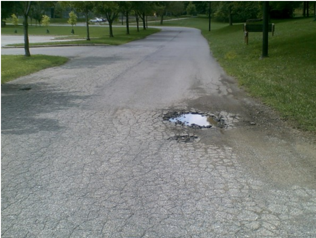
Photograph No. 6: High severity fatigue cracking and large pothole in access drive. Note area of patching or overlay at top of photograph.
