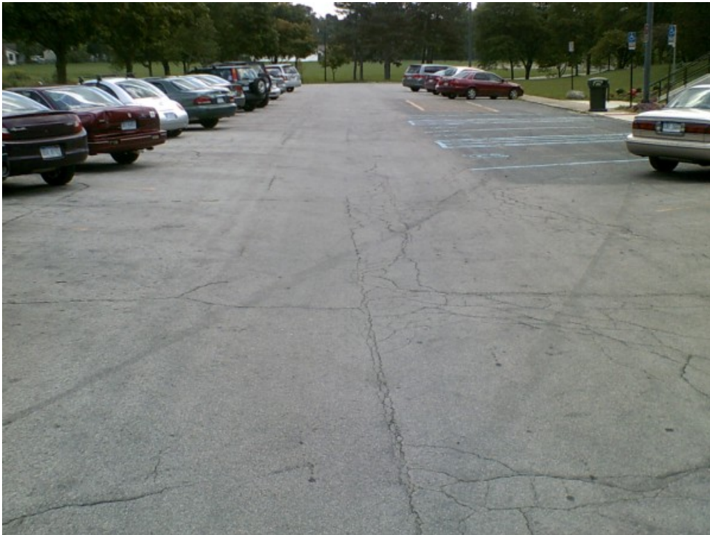
Photograph No. 2: Moderate severity longitudinal and fatigue cracking in north parking lot.
