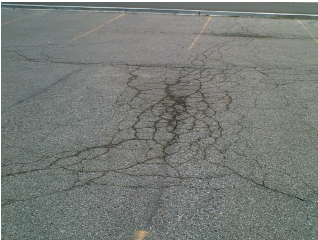
Photograph No. 10: High severity fatigue cracking.
