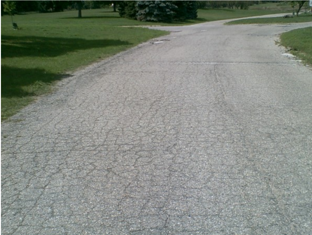
Photograph No. 5: High severity fatigue cracking in north access drive.
