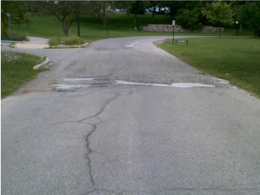
Photograph No. 17: Moderate to high severity transverse cracking and fatigue cracking with ponding water in access drive.
