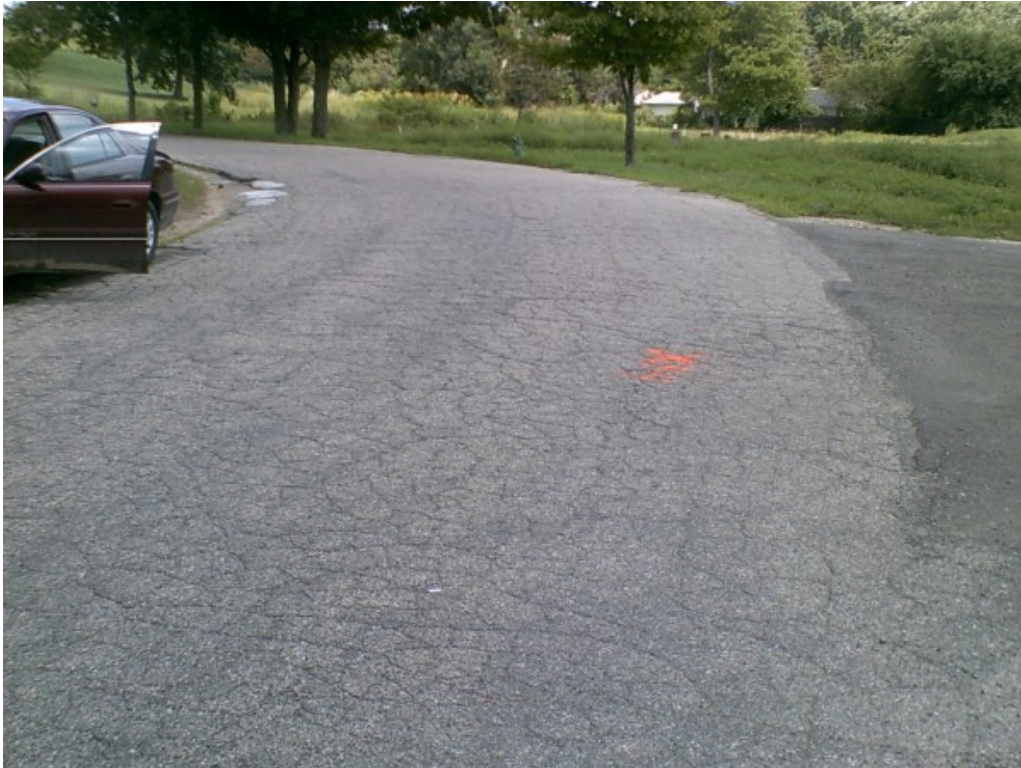
Photograph No. 7: High severity fatigue cracking in access drive. Note no curbs are present.
