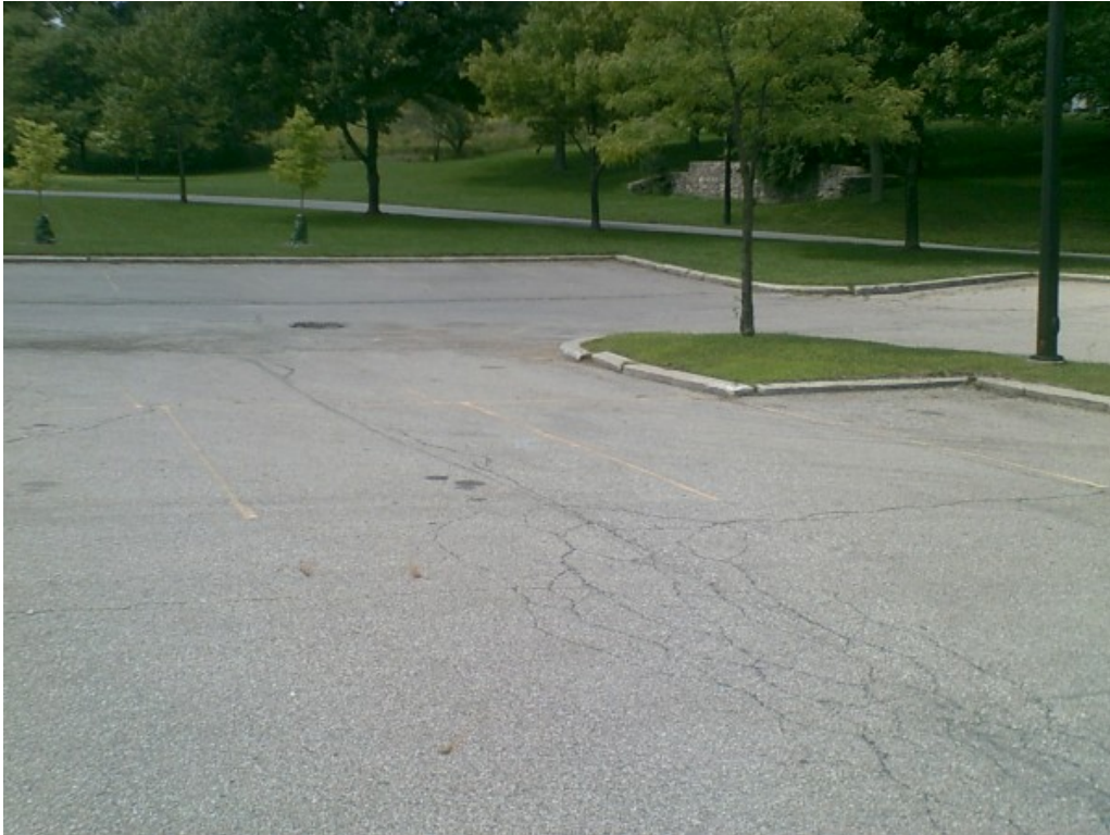
Photograph No. 9: Low to moderate severity fatigue cracking in south parking lot. Note curbs are constructed of concrete parking blocks.
