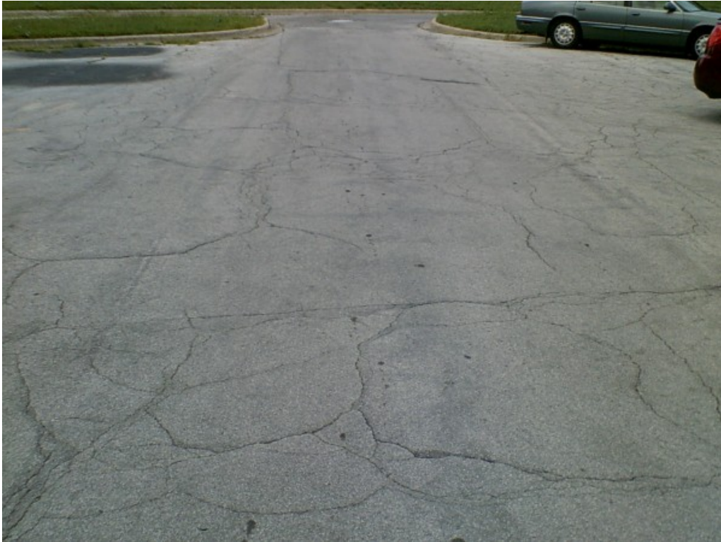
Photograph No. 1: Moderate to high severity fatigue cracking in north parking lot.
