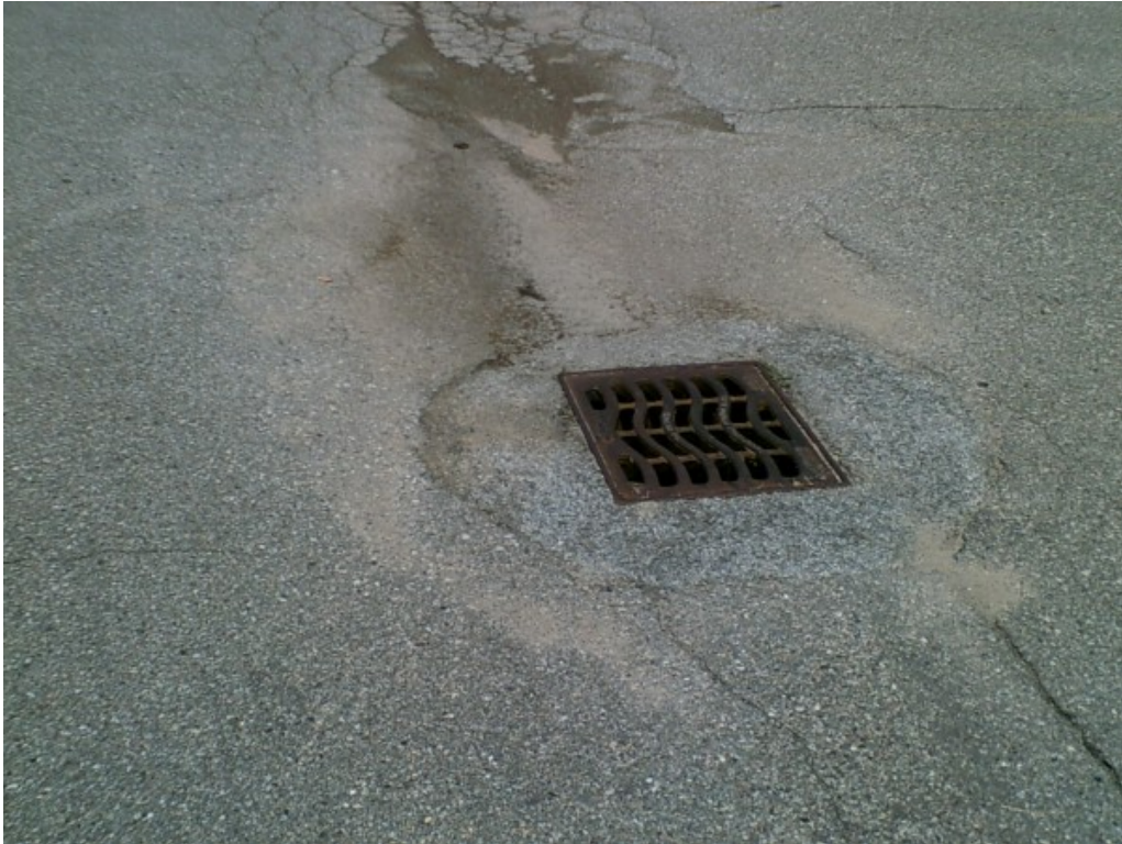
Photograph No. 11: Moderate severity fatigue cracking and evidence of previous ponding. It appears previous rehabilitation may have been performed around catch basin.
