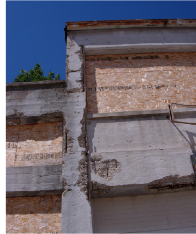
Concrete spalling on west concrete frame
