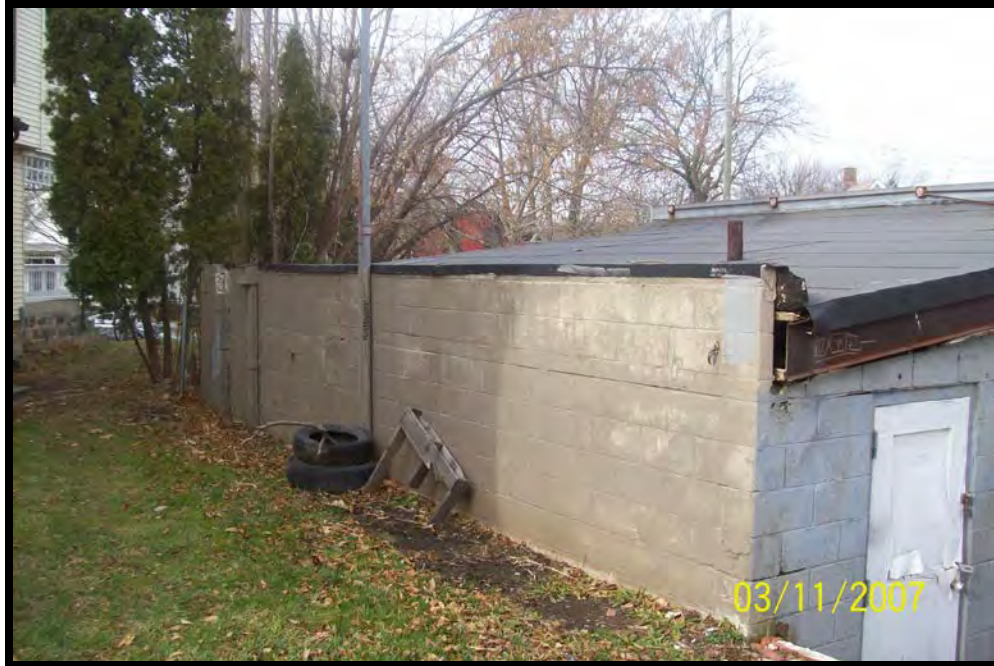
PHOTOGRAPH NO. 3: SUBJECT PROPERTY SOUTHERN PORTION OF THE SUBJECT BUILDING (VENT PIPES ALONG WALL)
