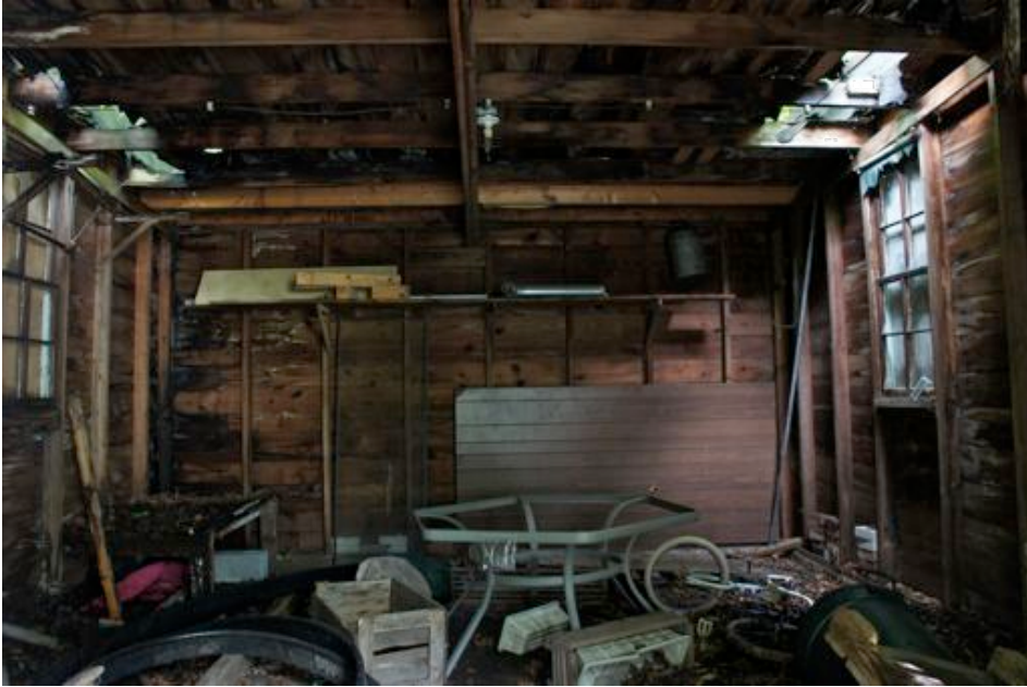
LEFT: photo of garage interior showing present deteriorated state
