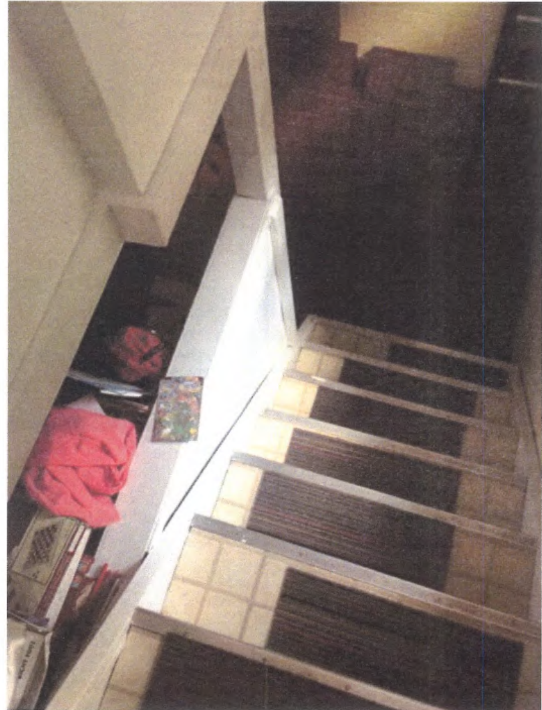
EXISTING BASEMENT STAIR (EXTERIOR WALL AT BTM OF STAIR TO BE FURRED OUT 5")
