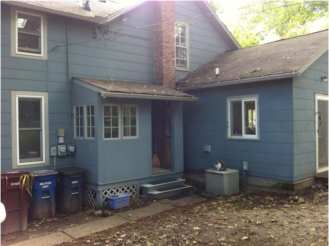
Photo 2. Shows slider window on previous kitchen addition that we will approximate for the new porch.
