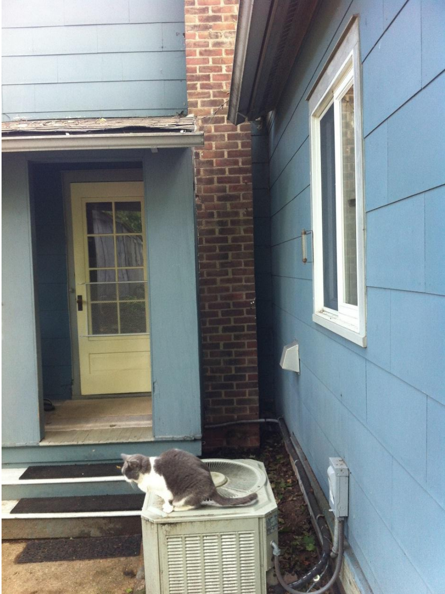
Photo 5. Shows gap between current porch roof and kitchen roof. This gap will be closed with new porch and rainwater will be routed away from this corner.
