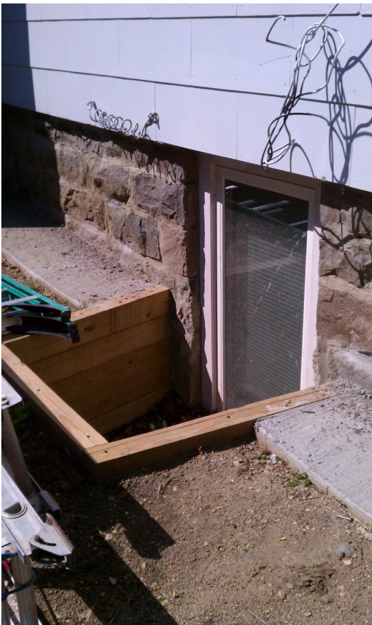
Example of installed egress window
