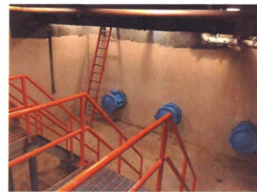
UV in an existing pump room inside the plant
