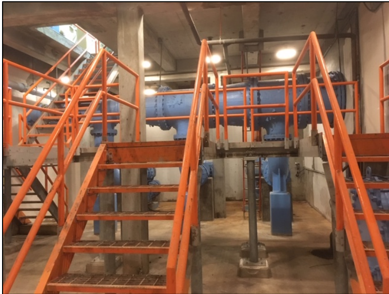
Figure 5. Transfer Pump 4–6 Room
