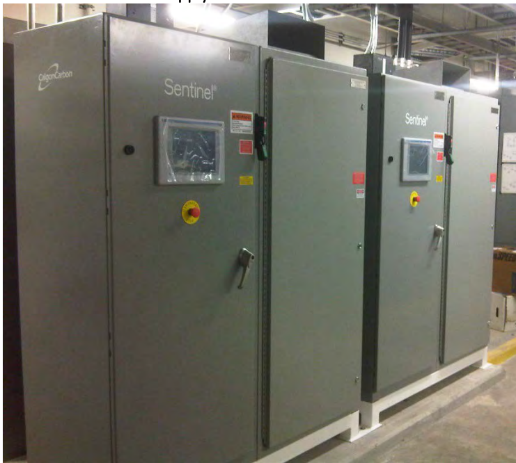
Exhibit 15. UV Power Supply Units
