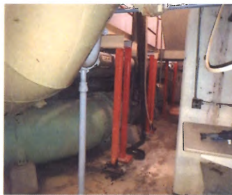
UV in existing pipes inside the plant
