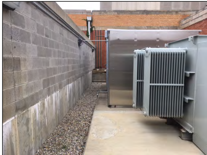
Figure 16. Screen Wall Electrical Equipment
