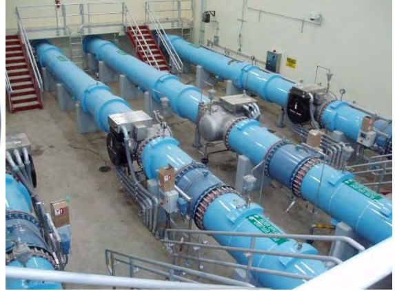
Exhibit 14. Water Plant UV Installation
