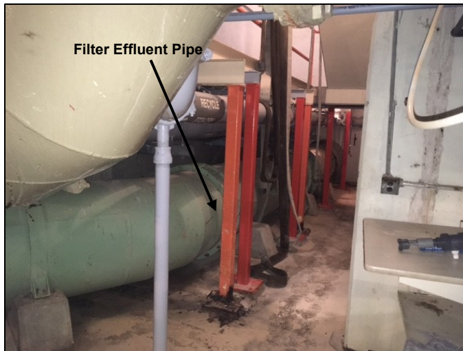
Figure 4. Filter 21–26 Effluent Pipe
