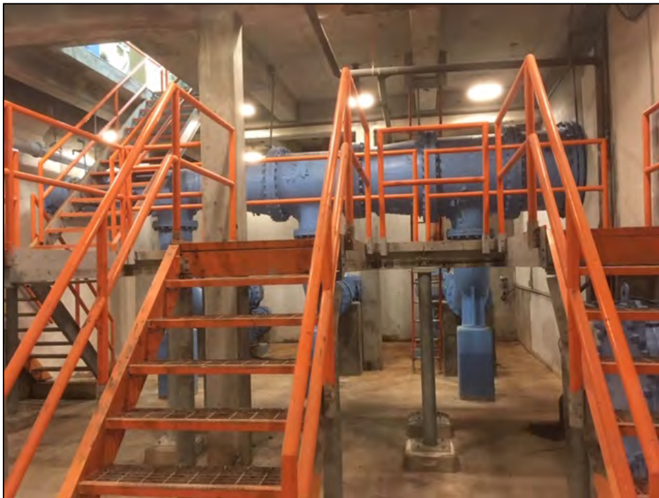
Figure 2. Transfer Pump 4–6 Room
