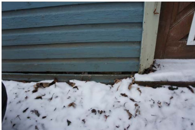
shed lower plate and siding buried below grade
