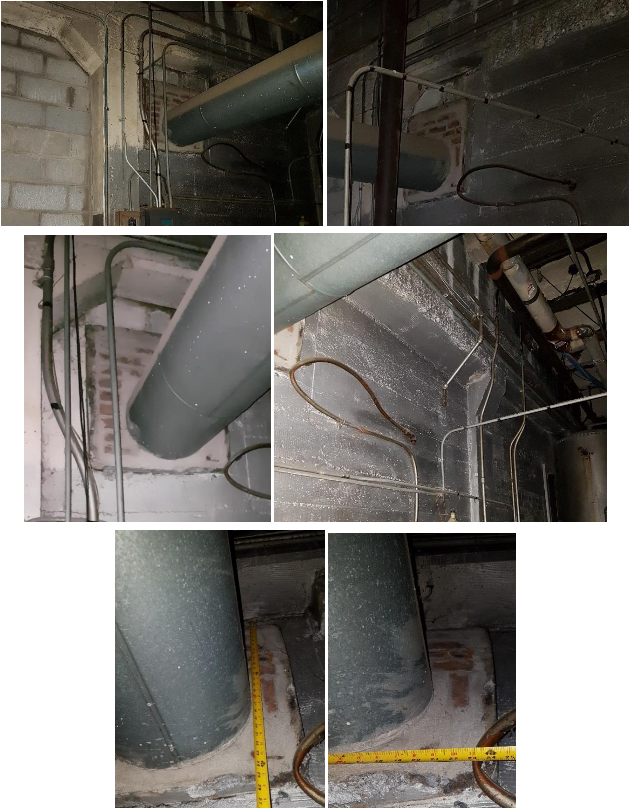
Photoset 5: Extension of the concrete beam end to the inside of the adjacent building.
