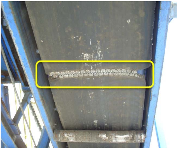
Lacing is damaged. Belt is torn.
