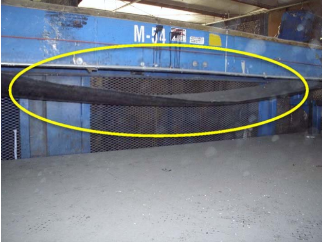
Tensioning is off, belt is not supported by any rollers.
