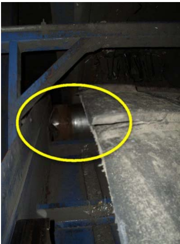
Belt tracking and tensioning completely off to the right.
