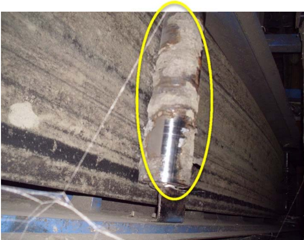
Return rollers are worn, replacement required.
