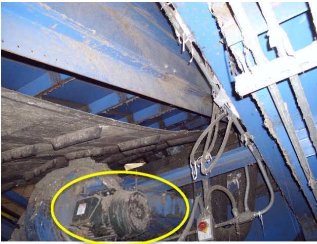
Gearmotor is leaking and needs to be replaced.
