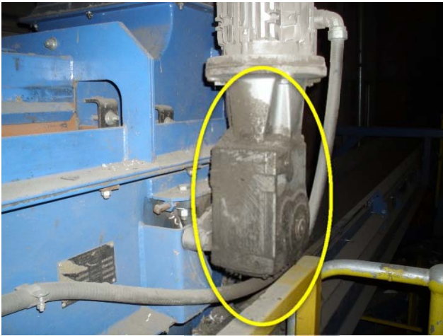
Gearmotor is leaking, replacement required.
