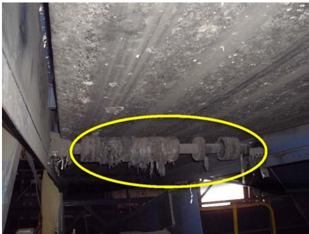
Return rollers are wrapped and worn, replacement required.
