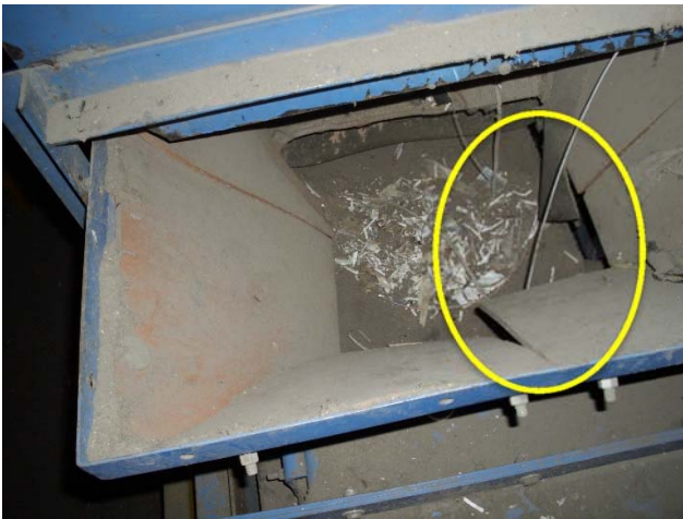
Liners need to be replaced.
