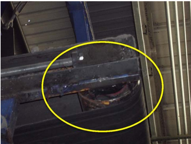
Picture shows severely worn pulleys and bearings.
