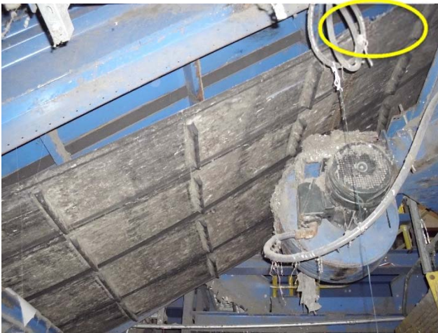
Belt is torn and needs to be replaced. Tensioning is lacking.
