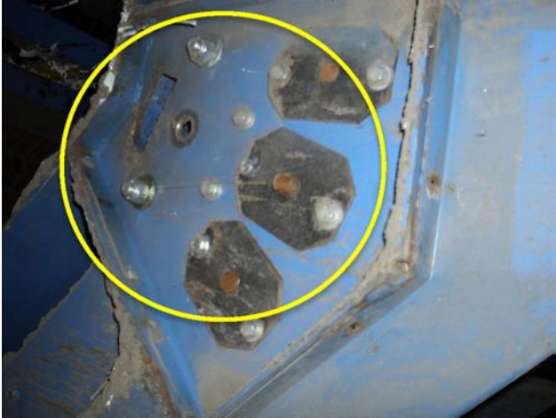
Return rollers omitted, replacement required.
