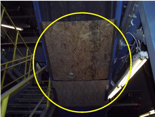
Plywood installed as belly pans, removal required.
