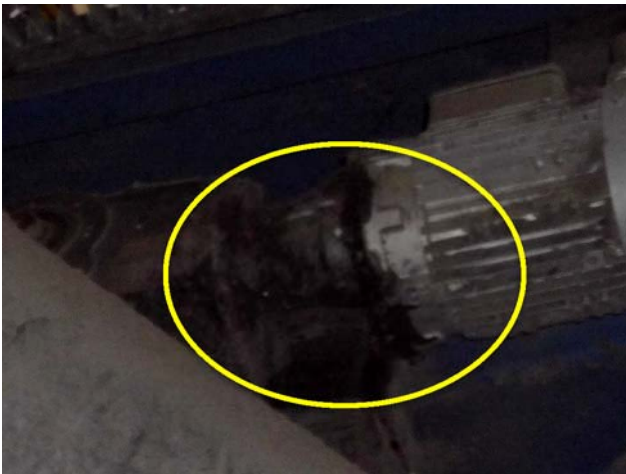
Gearmotor is leaking.
