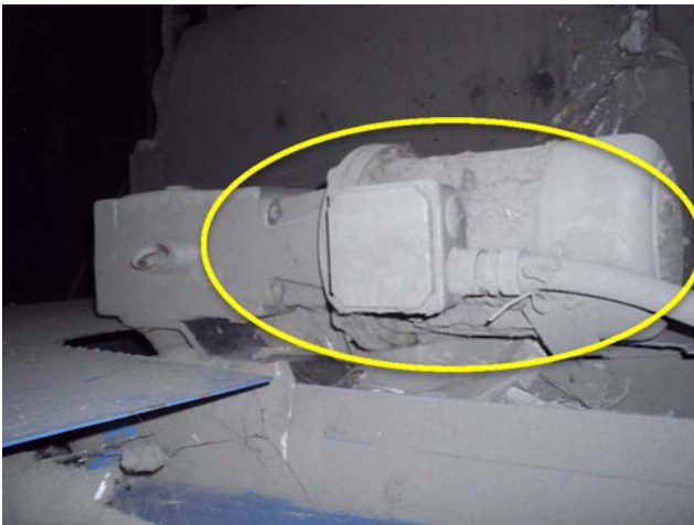
Motor is filled dust and surrounded by debris, replacement required.
