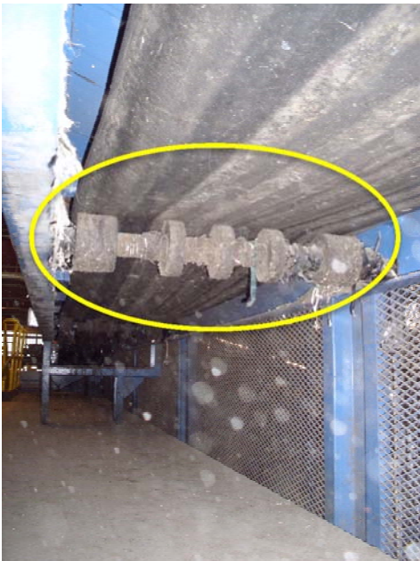
Return rollers are worn, replacement required.
