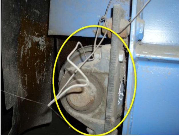
Bearing is worn, tracking of belt veers to the right, replacement required.
