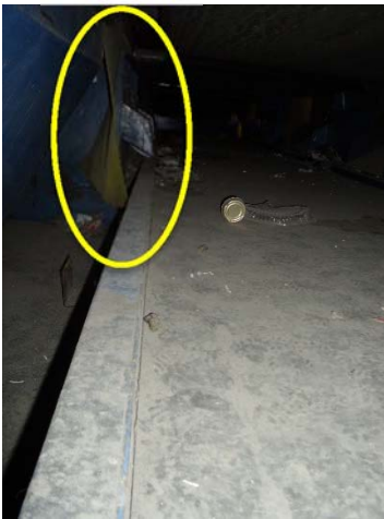
Guarding needs to be repaired/replaced.
