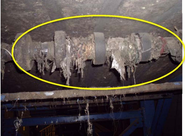
Return rollers are worn, replacement required.
