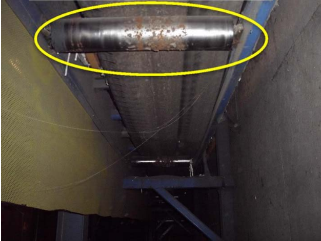
Return rollers are worn, replacement required.
