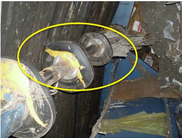
Return rollers are worn and needs to be replaced.
