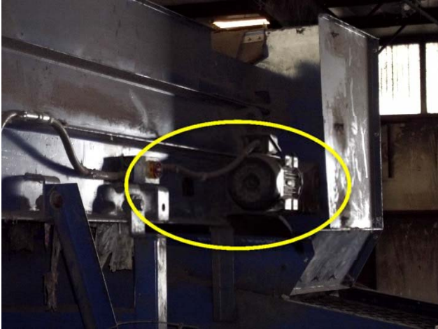
Gearmotor is leaking, replacement needed.
