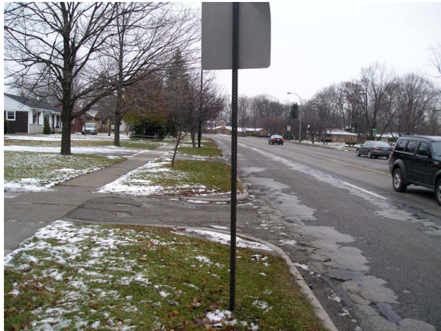
W. Stadium 2009 Condition "Poor"
