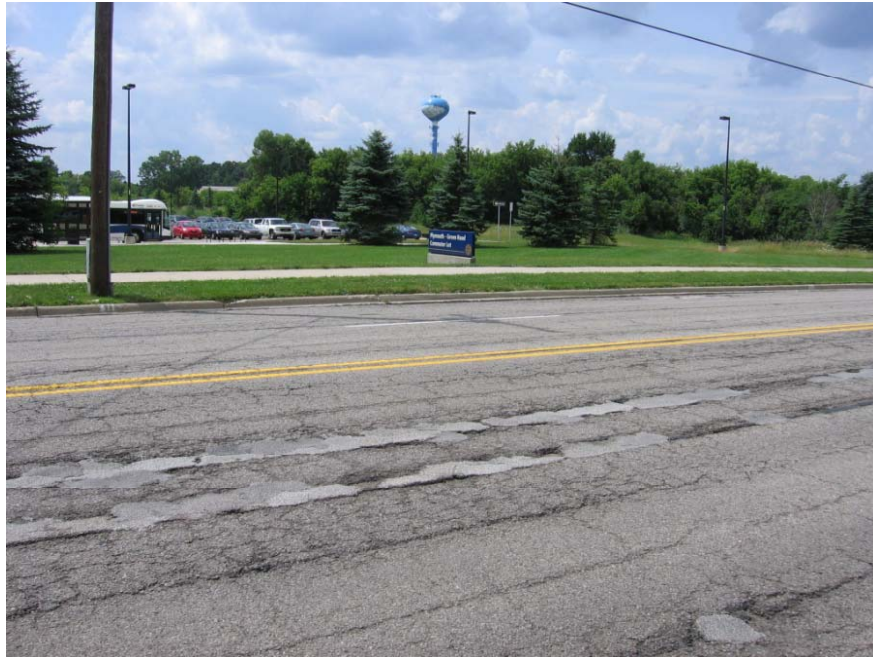
Green Rd 2009 Condition "Poor"
