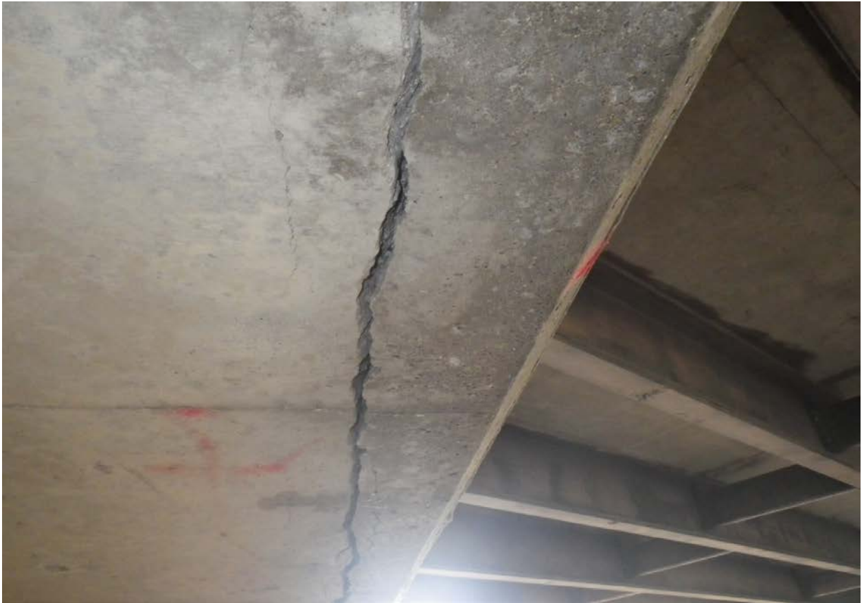
Figure 13 Cracked Pier Cap (North Pier (Pier 2))
