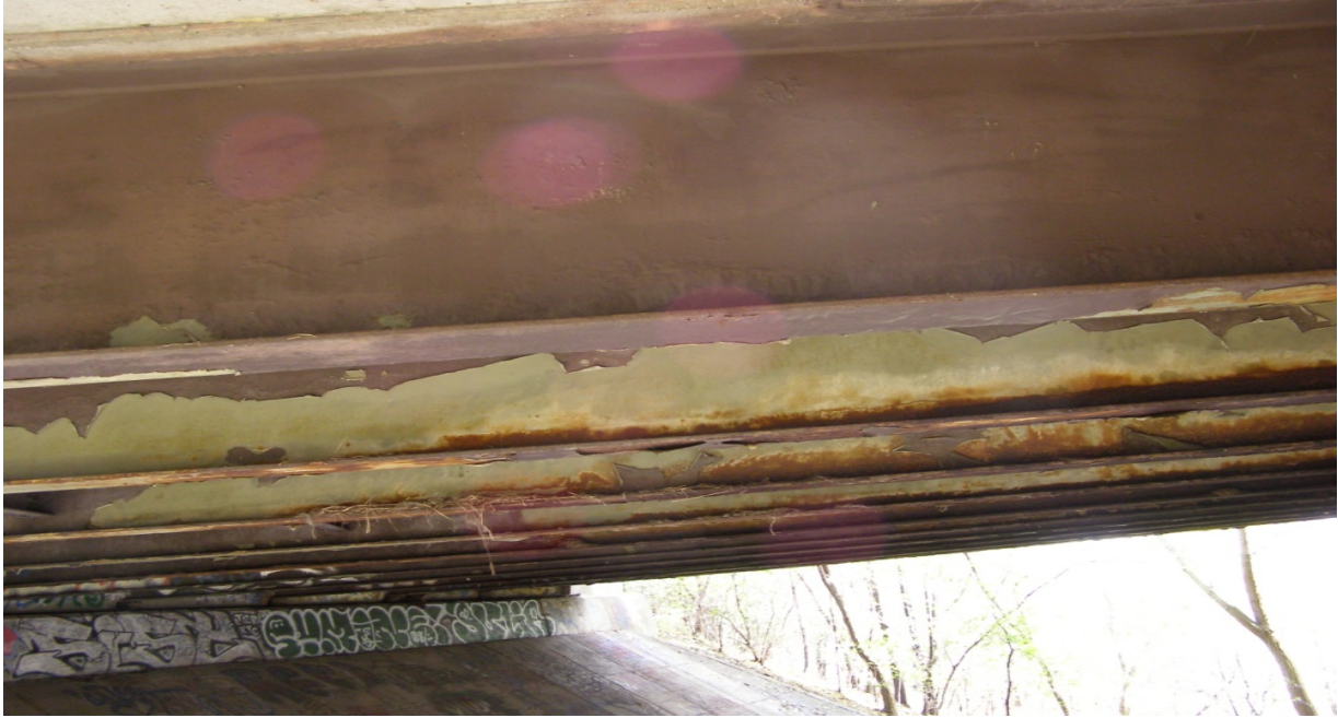
Figure 12 Paint Failures at bottom flange of beams
