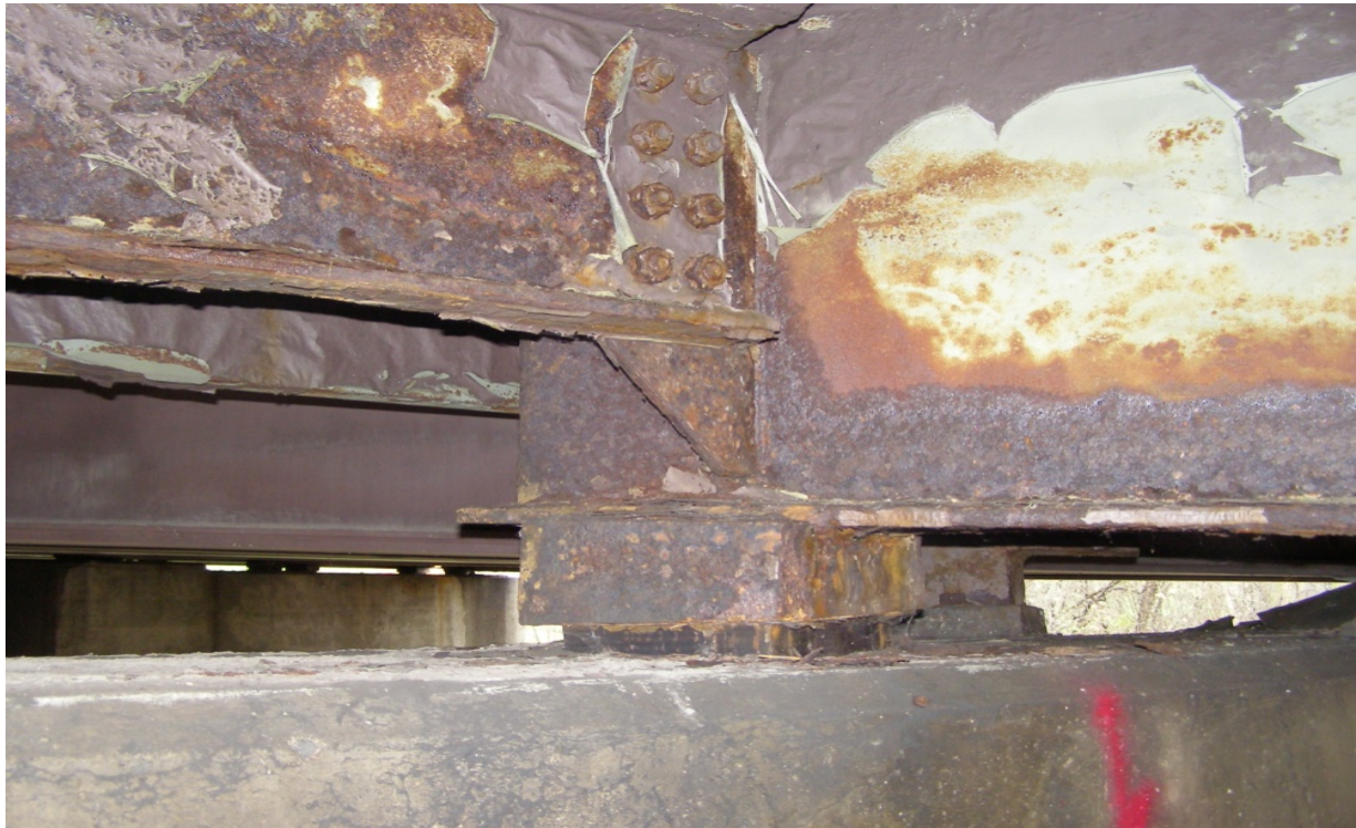
Figure 10 End Diaphragm and Beam End Surface Rusting and Paint Failure, Pier 2
