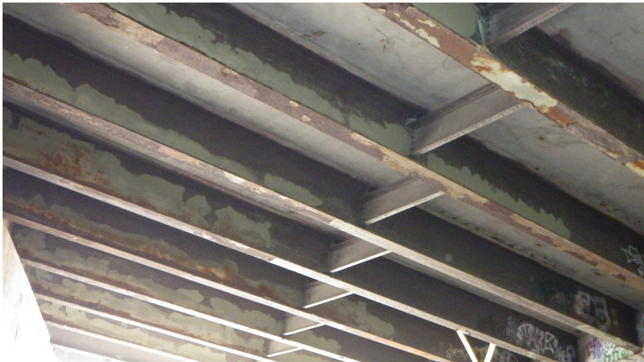
Figure 11 Typical Paint Failure
