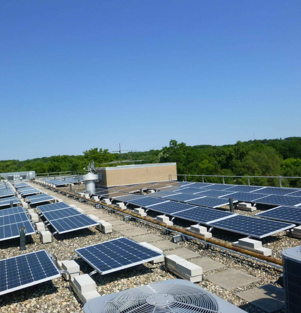
Solar on Miller Rooftop
