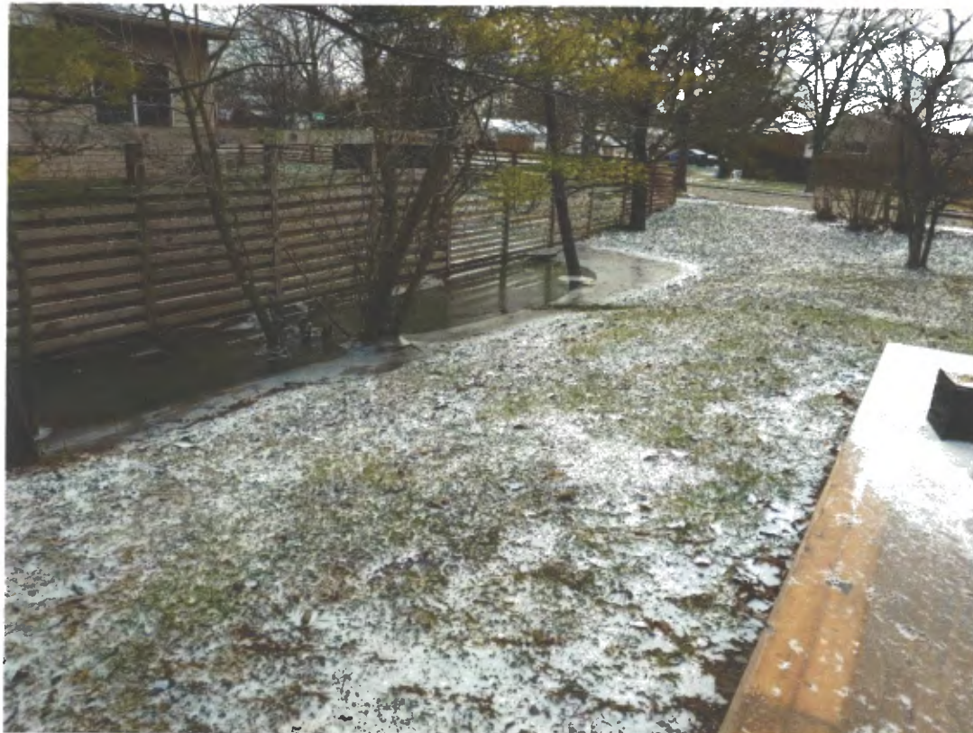
4) View Southeast from deck, showing the large depression on the eastern side of the yard and the ponding from ½" of rain January 11-12, 2020.
