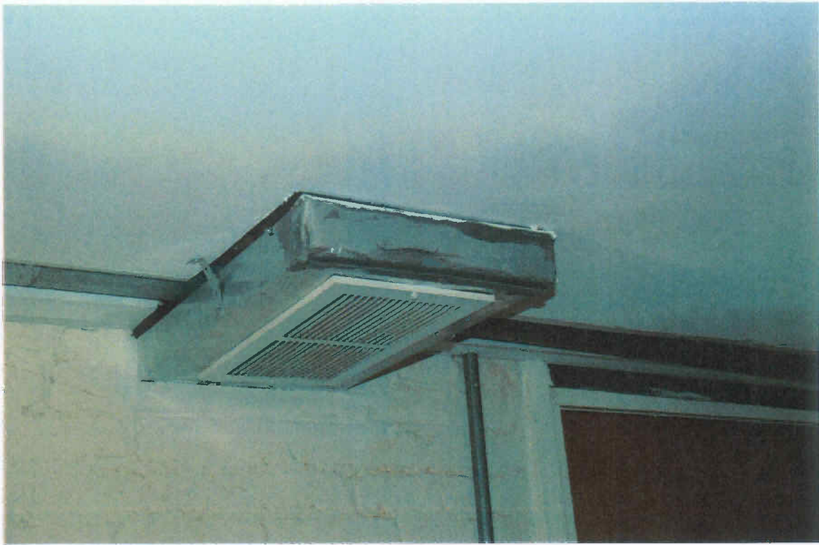
Room 13 Duct C
