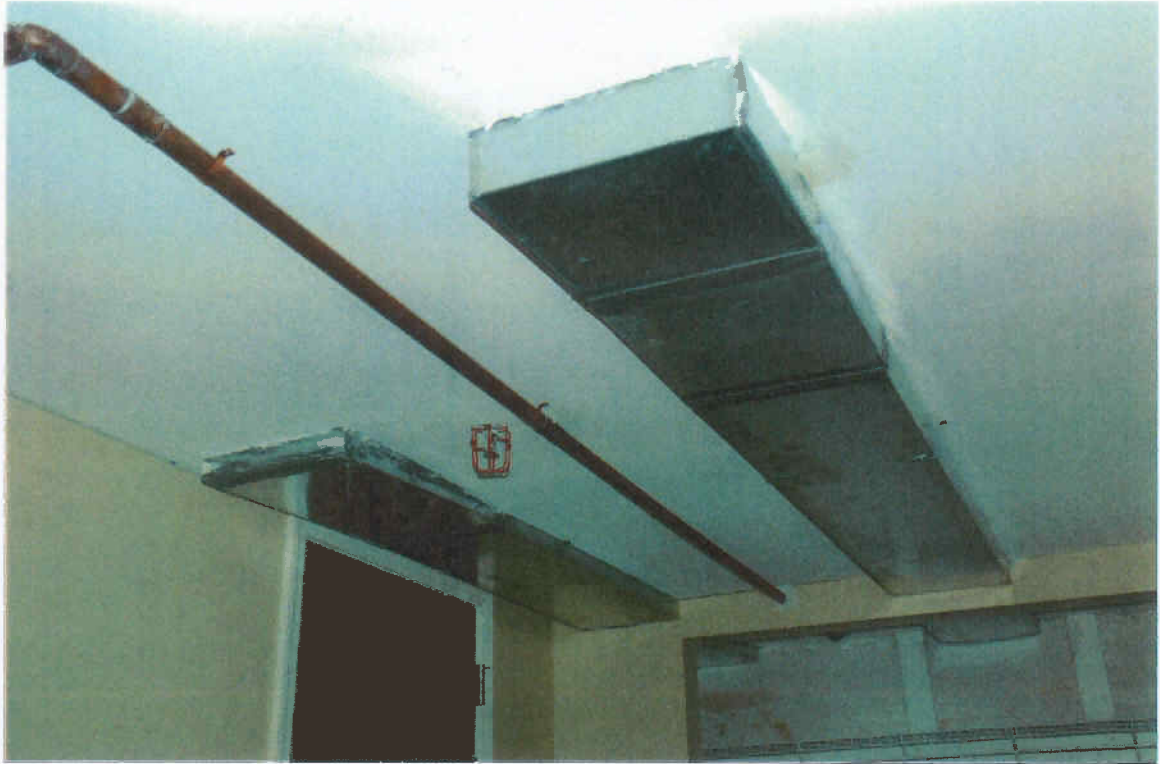
Room 12 Sprinkler pipe and Ducts A & B
