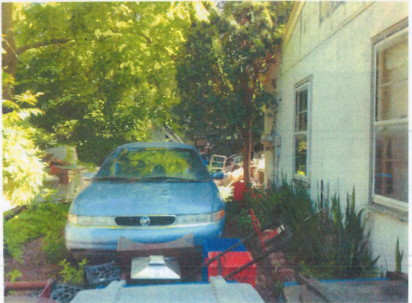
Partially collapsed garage behind car
