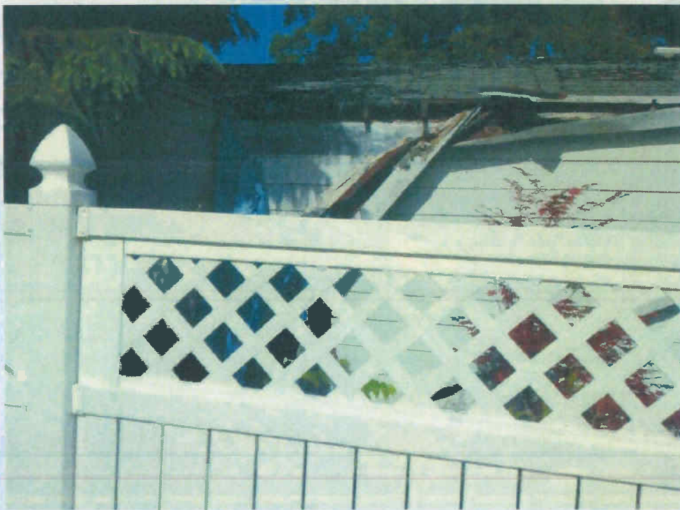
rear addition in disrepair
