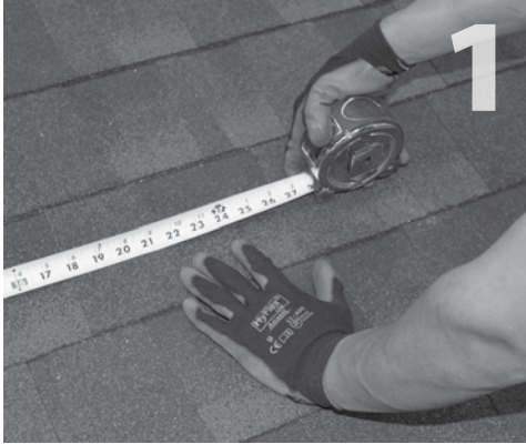
1 Locate, choose, and mark centers of rafters to be mounted. Select the courses of shingles where mounts will be placed.
