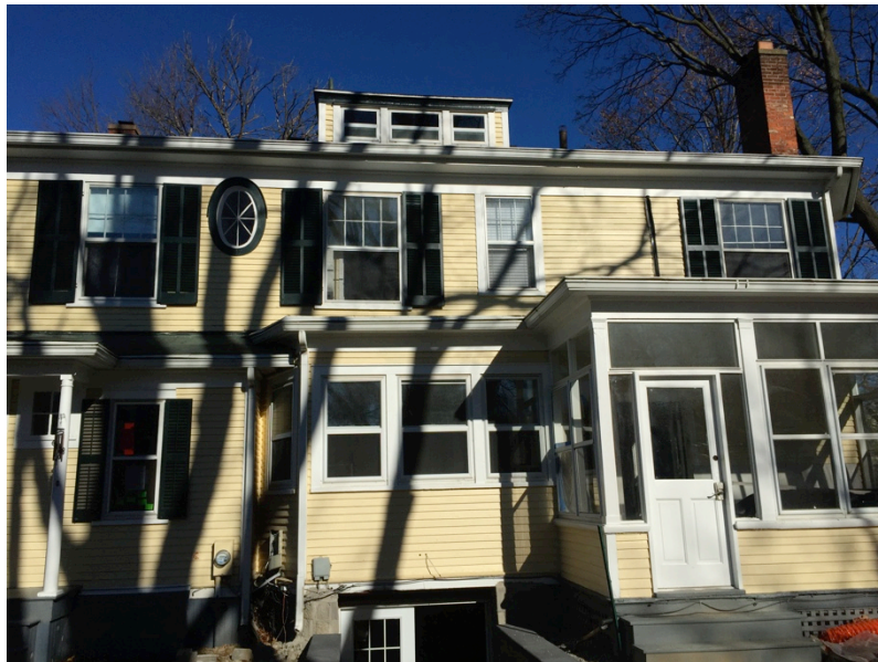
Mini-split line-set above the back porch.
