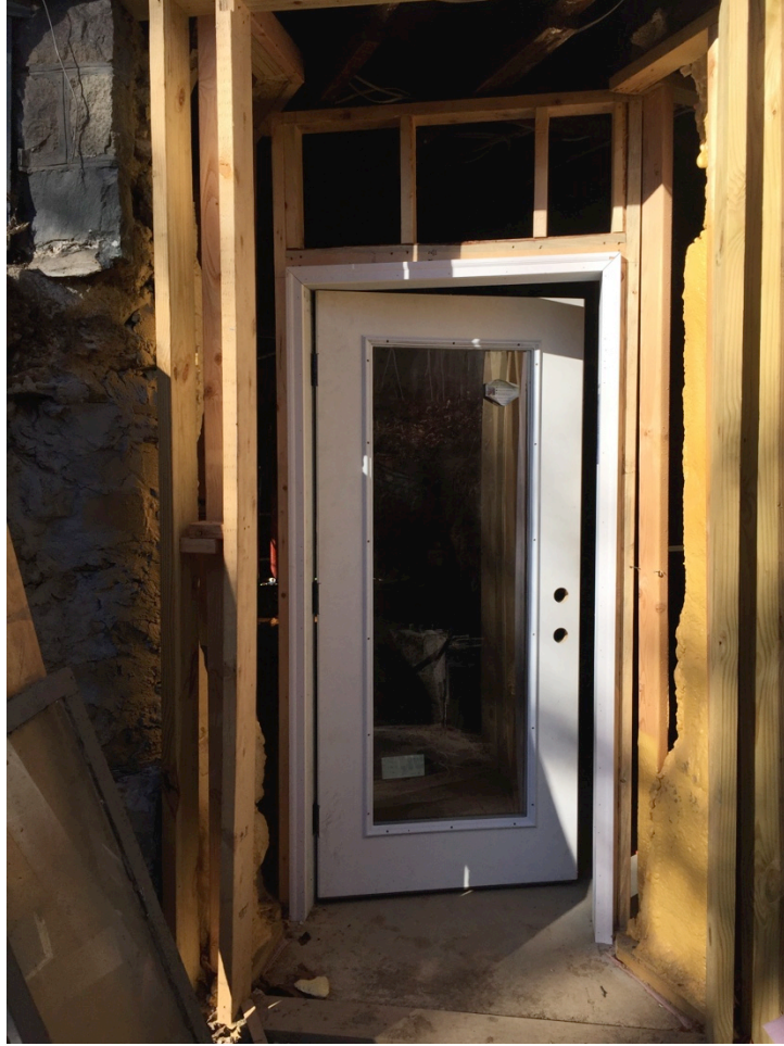
A Jeld-Wen full light door is being installed at the east entrance.
